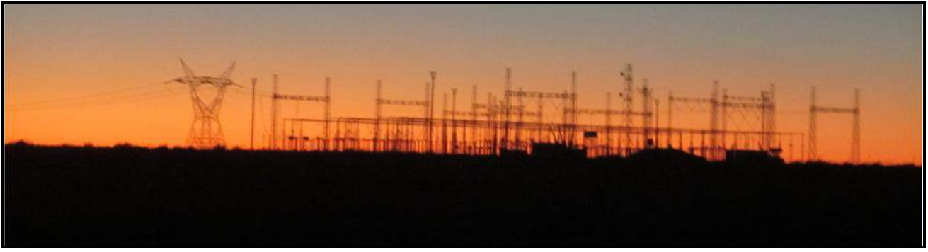
Figure 21: Evening view of the large Eskom substation located some 16 km south of the proposed project.
