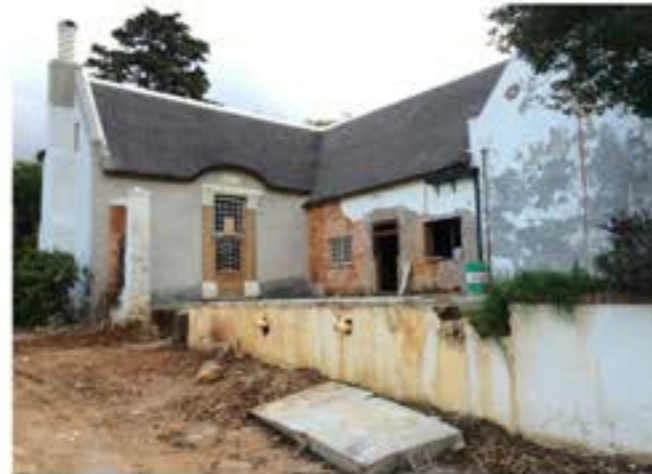
Image 04: Adjusted east façade openings (Jan 2014 approval) and pergola location in front of blank gable.
