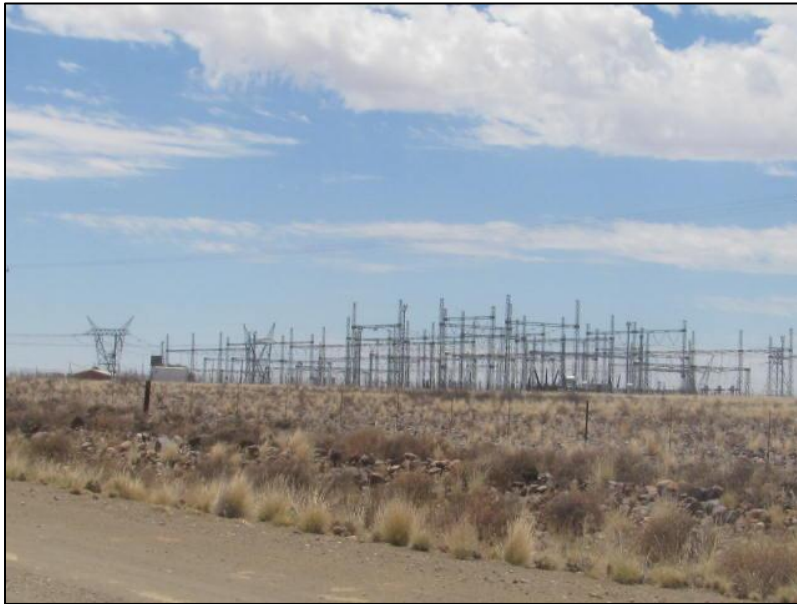
Figure 5-7: Aries substation 1 km south of the study area
