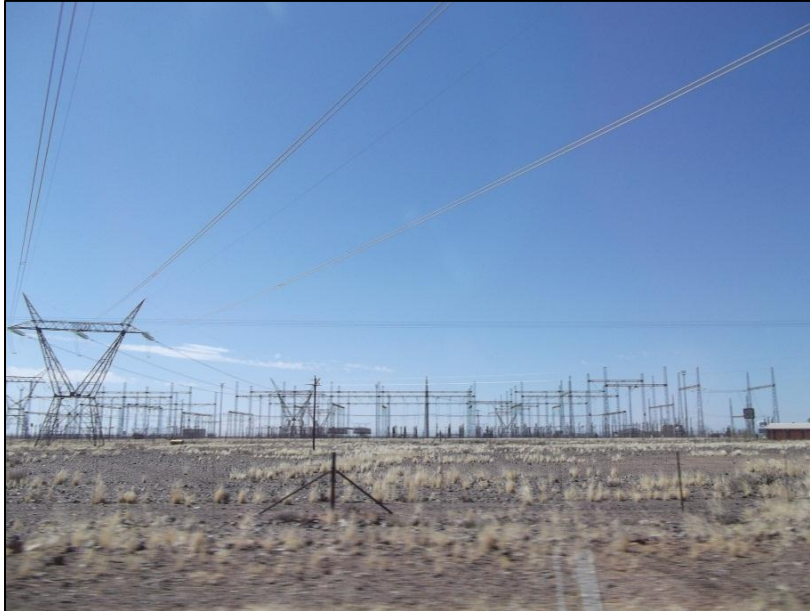
Figure 5-2: Aries substation and 400 kV CRS transmission lines to the south of the project site
