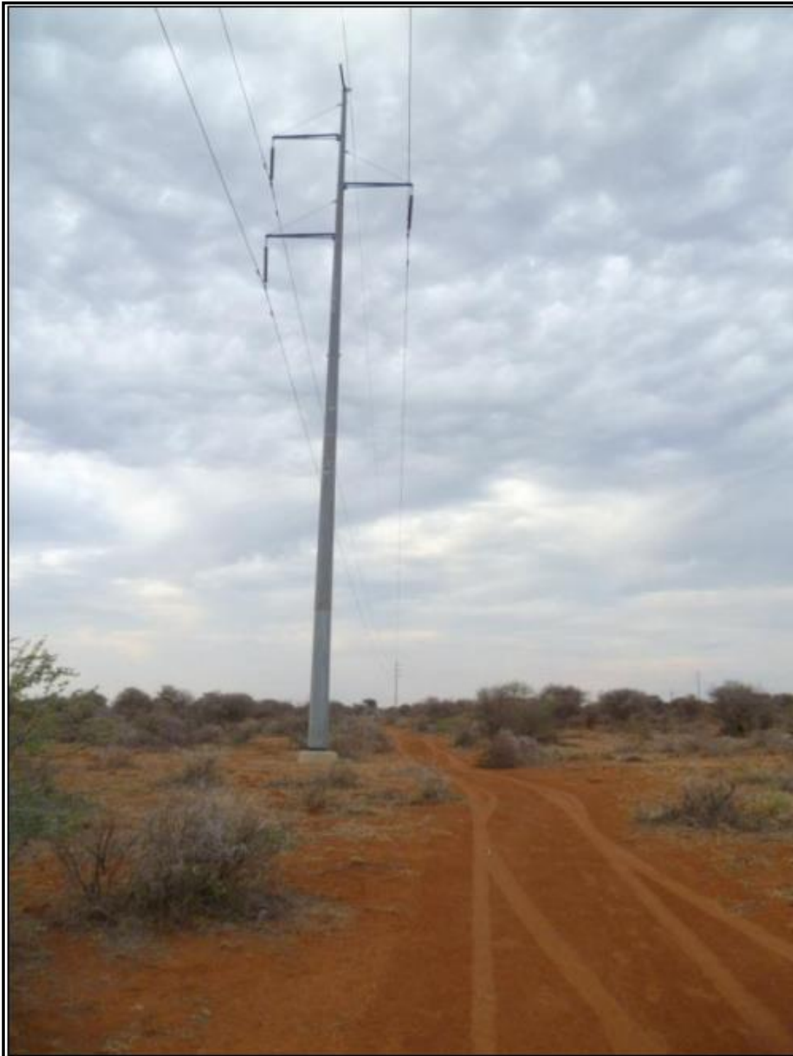
Plate 2: Photograph of a Typical 132 kV Powerline
