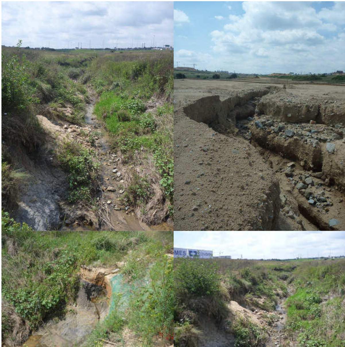
Figure 3: Photographs indicating severe erosion and degradation in the watercourse prior to rehabilitation.
