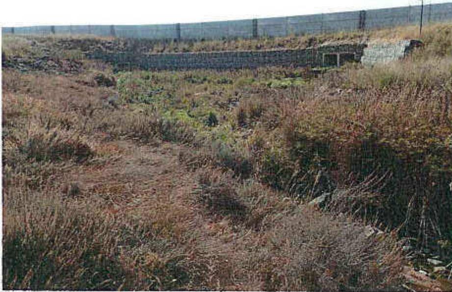
Figure 1 Storm water inlets and concentrated flows of water entering the lower portion of the watercourse
