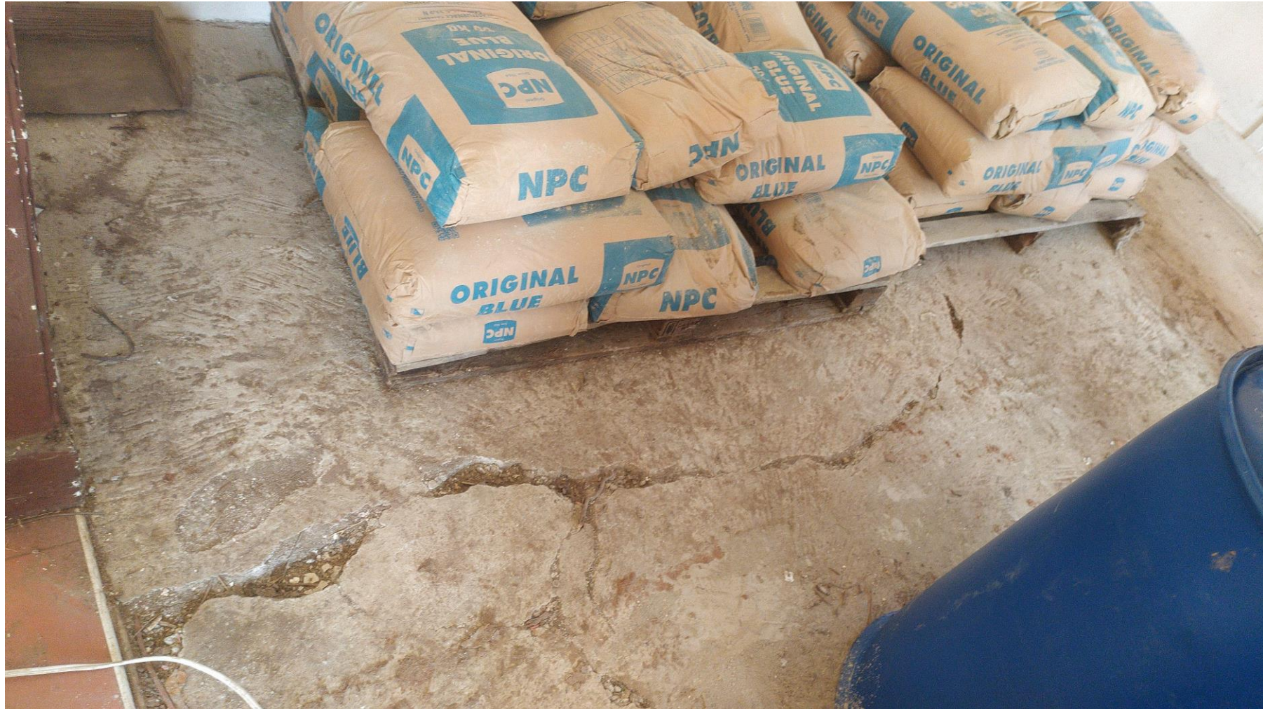
CRACKED CONCRETE FLOOR SLABS
