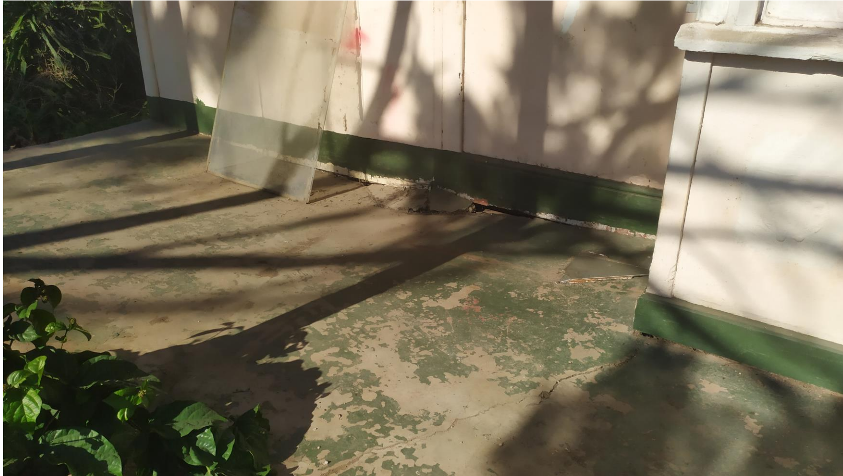
FRONT STOEP SHOWING THE CRACKED CONCRETE BASE
