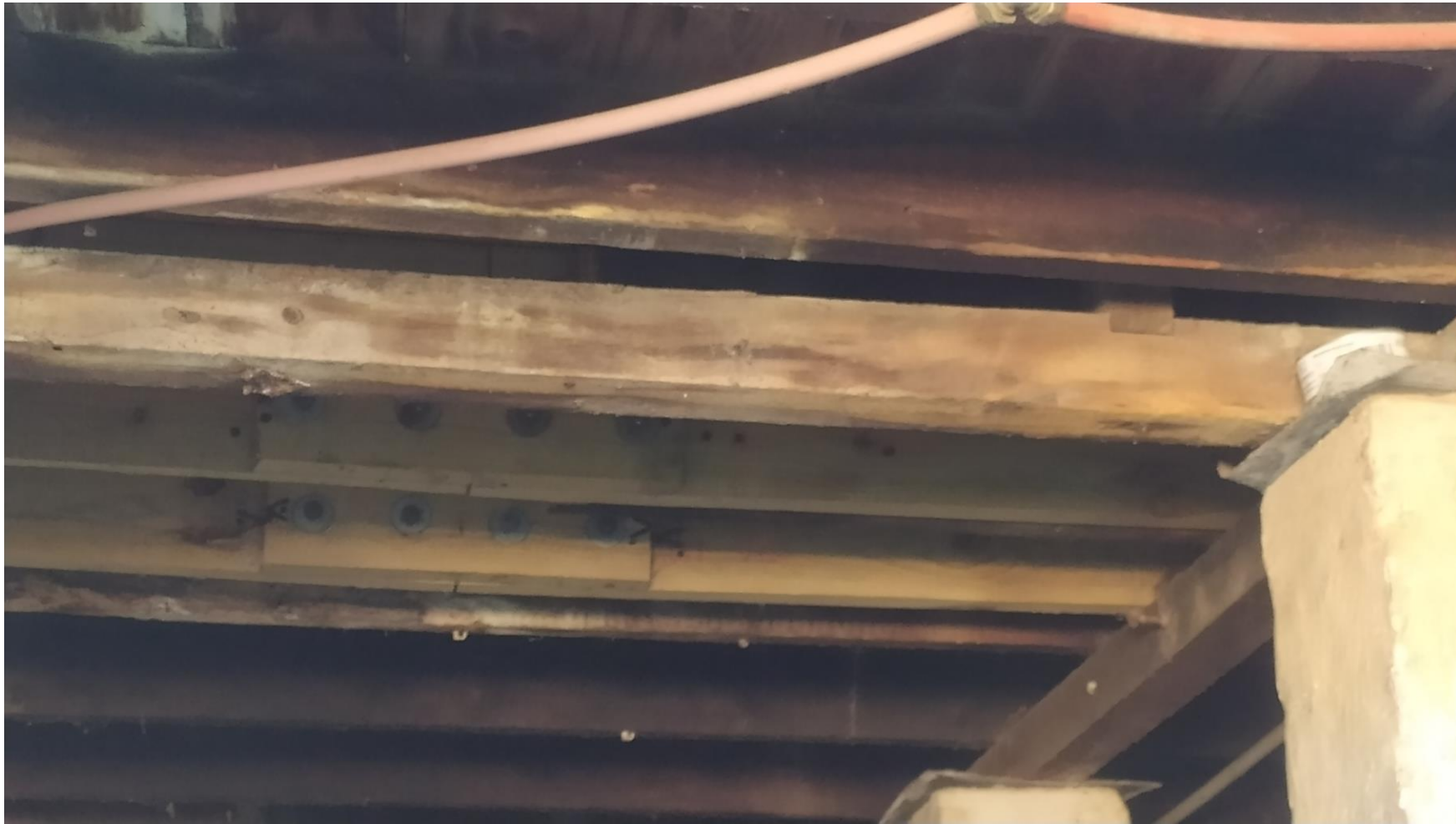
THE DAMPNESS IN THE CRAWL SPACE HAS STRUCTURALLY AFFECTED THE TIMBER SUPPORTS FOR THE FLOOR AND THE TIMBER IS AFFECTED WITH WOOD BORERS
