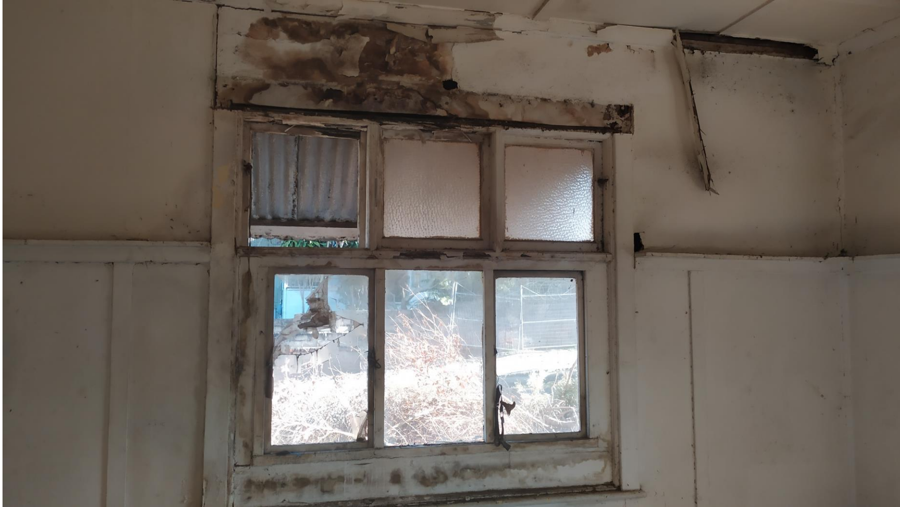
DAMPNESS FROM THE ROOF HAS ENTERED THE HOUSE AFFECTING THE HEALTH AND SAFETY OF THE HABITANTS
