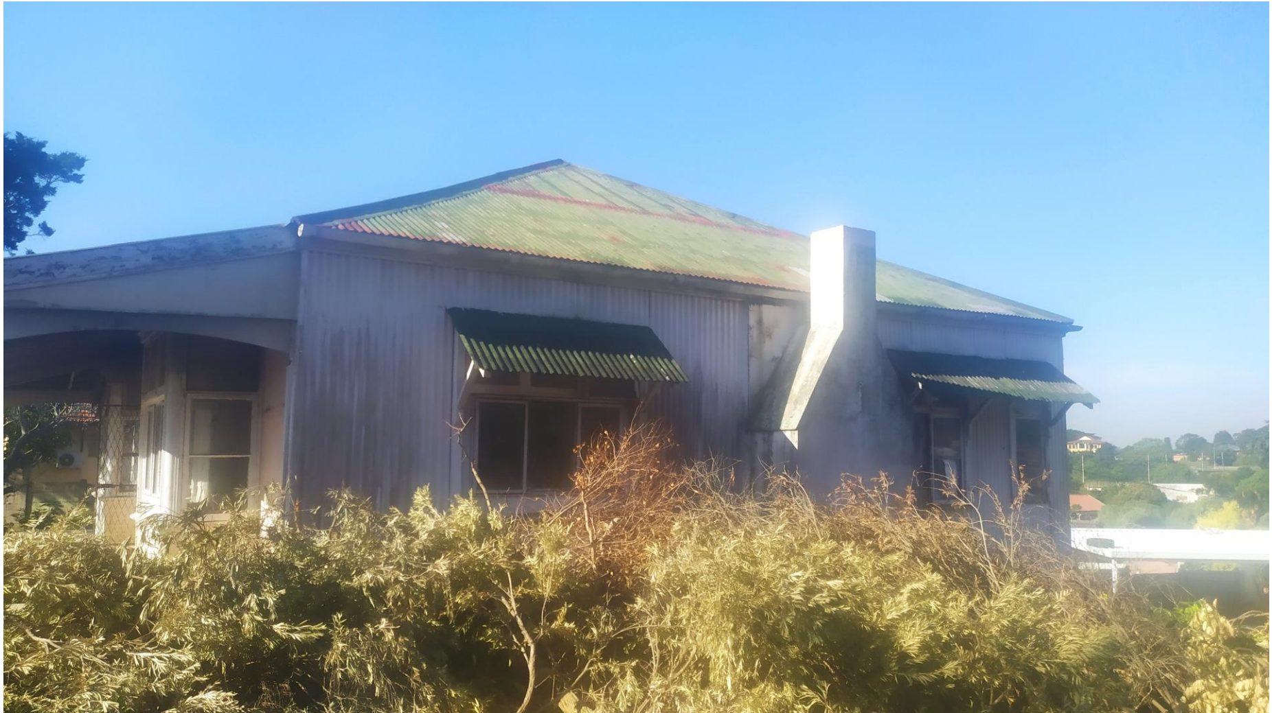
EXTERIOR FAÇADE- ILLUSTRATING TIN WALL STRUCTURE AND BROKEN AWNINGS
