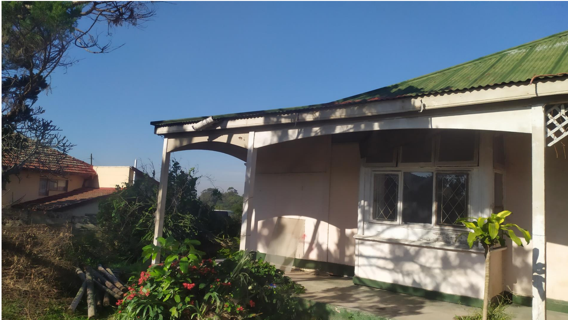
EXTERIOR FAÇADE- ILLUSTRATING TIN ROOF AND BROKEN GUTTERS
