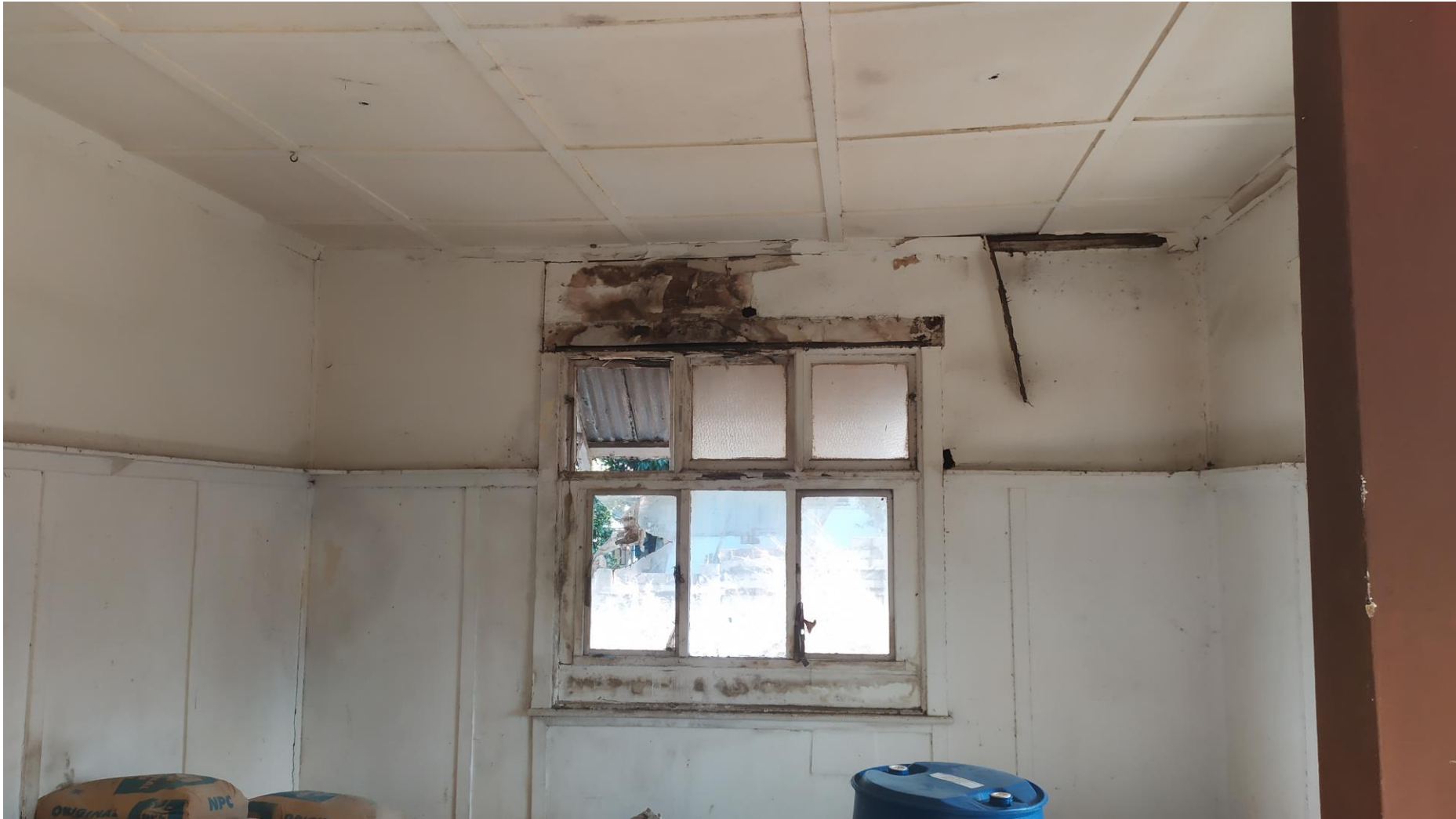
DAMPNESS FROM THE ROOF HAS ENTERED THE HOUSE AFFECTING THE HEALTH AND SAFETY OF THE HABITANTS
