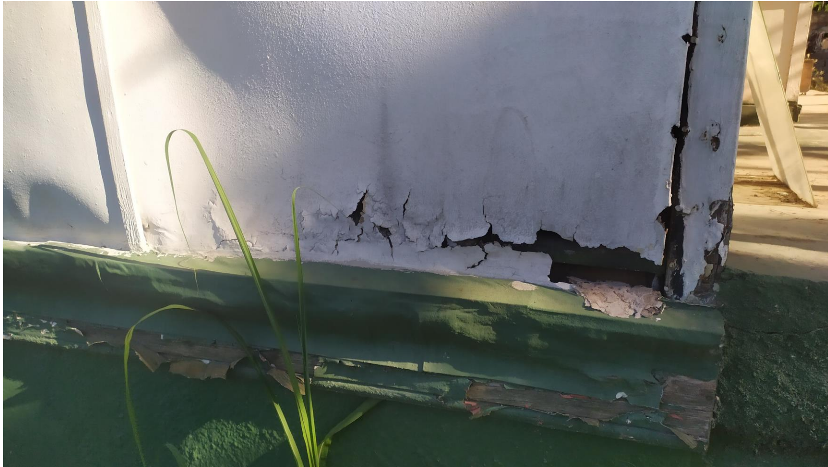
EXTERIOR FAÇADE- ILLUSTRATING TIN WALL STRUCTURE THAT IS ERODED AND TIMBER WALL SUPPORTS INFESTED WITH WOOD BORERS
