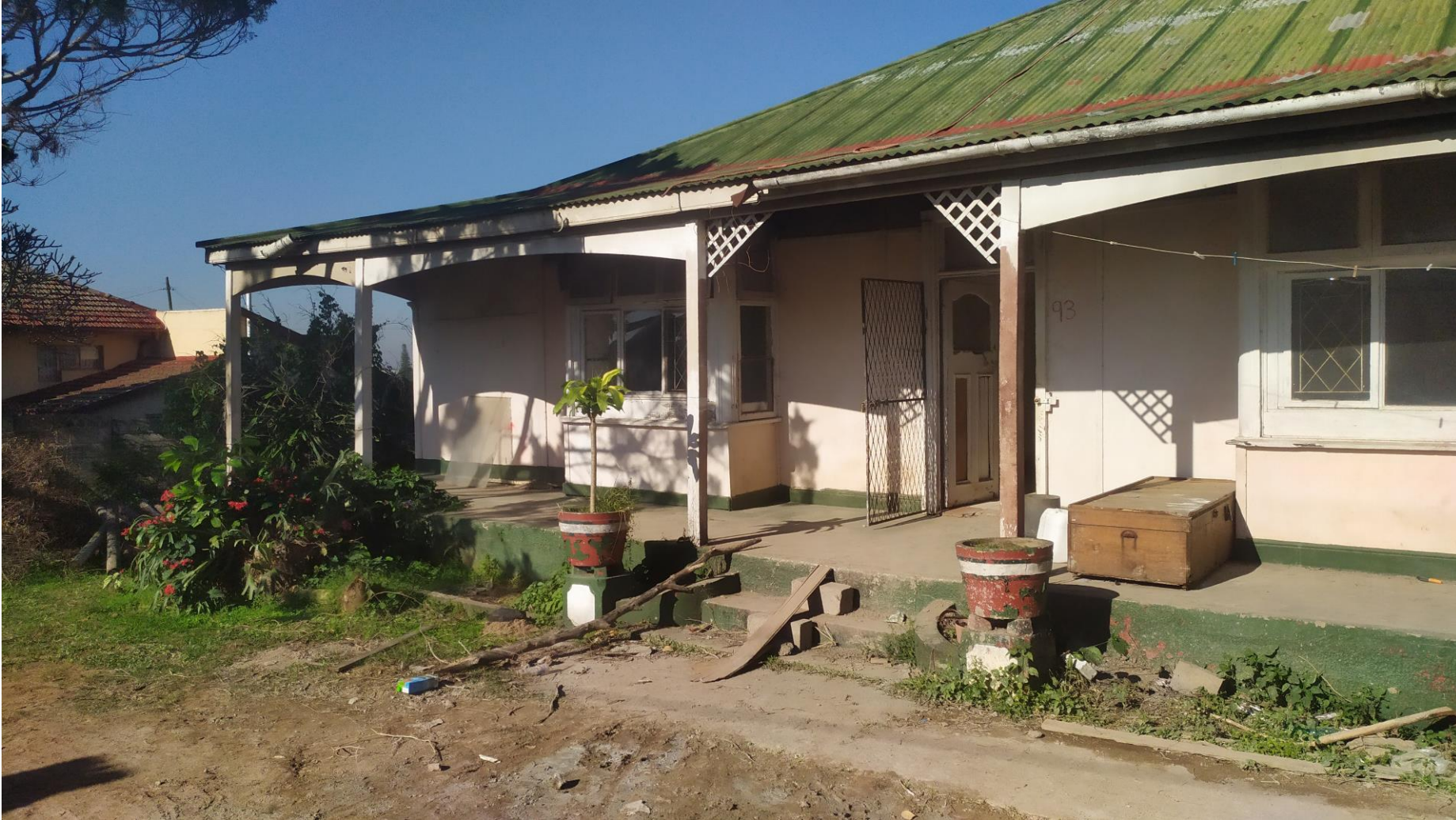
EXTERIOR FAÇADE- ILLUSTRATING TIN WALL STRUCTURE AND BROKEN AWNINGS
