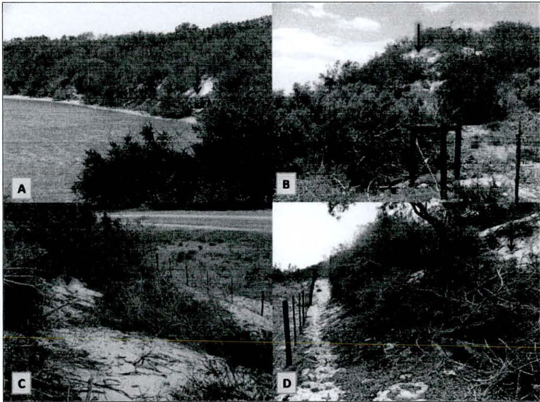
Photo 4: Dune area: (A) Erosion along river bank southwards of proposed activity; (B) Exposed dunes prone to slumping on eastern edge adjacent to rover; (C-D) Exposed base of dunes with inadequate topsoil and vegetation cover.
