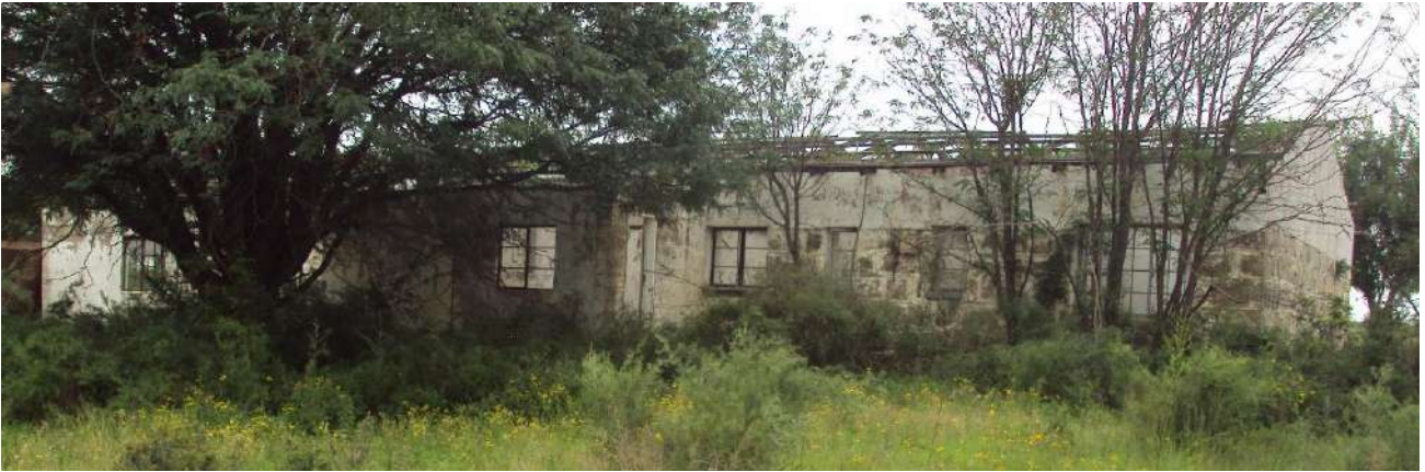
Figure 26: View of the front elevation of the main farmhouse, showing the overgrown and dense vegetation
