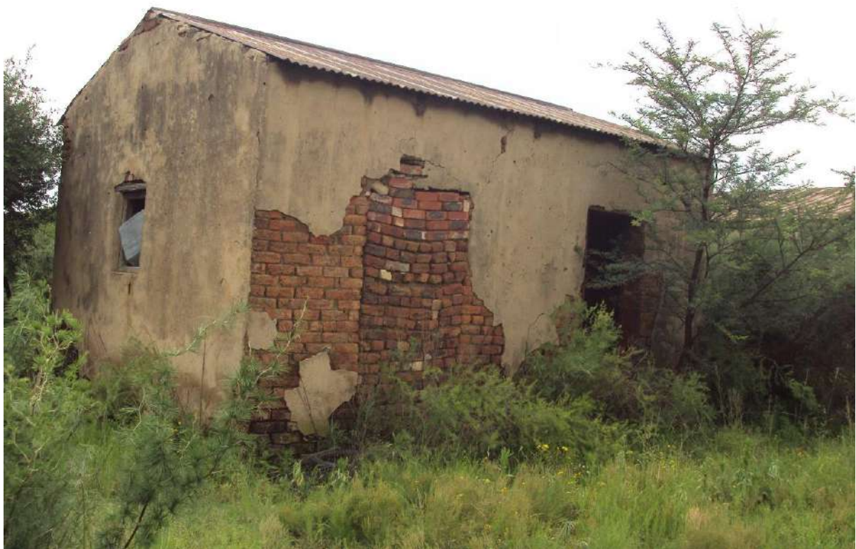
Figure 29: View of the historical structure adjacent to the barn, showing the old bricks and alterations
