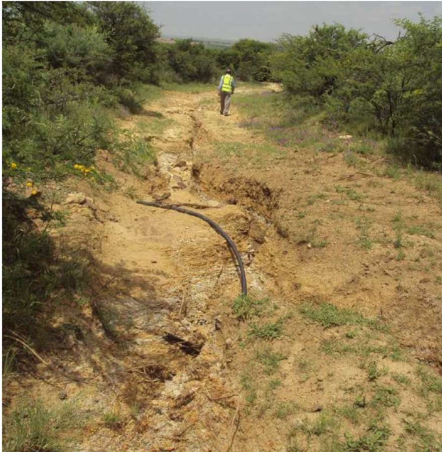
Figure 8: View of a heavily eroded farm road in the north-western section of the project footprint
