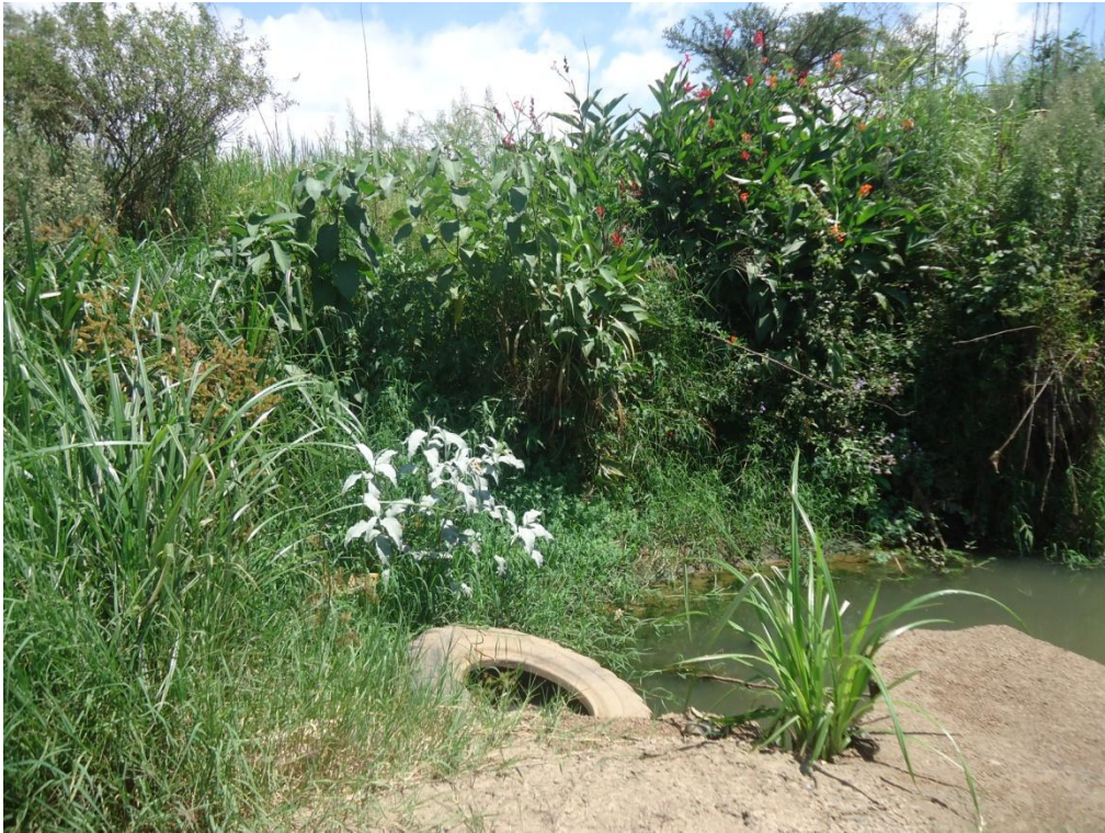
Immediate upstream side of existing bridge, note weeds, dumping, and cyperus.
