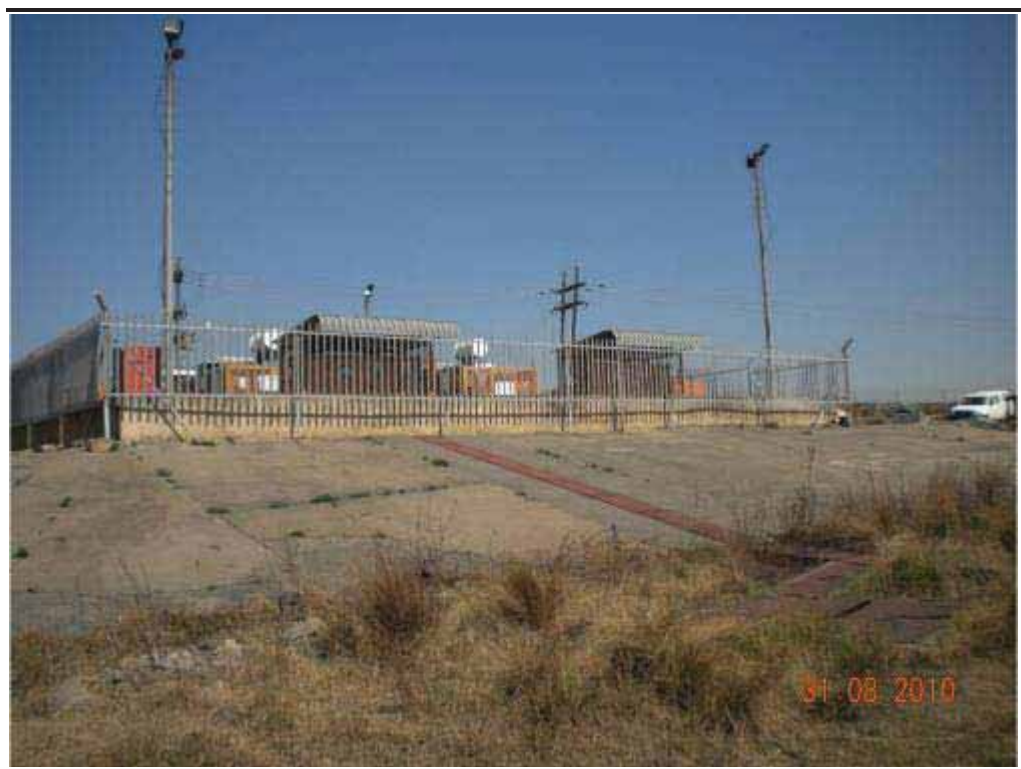
Figure 2.7 Typical Electrical Substation associated with a Main Mine Adit
