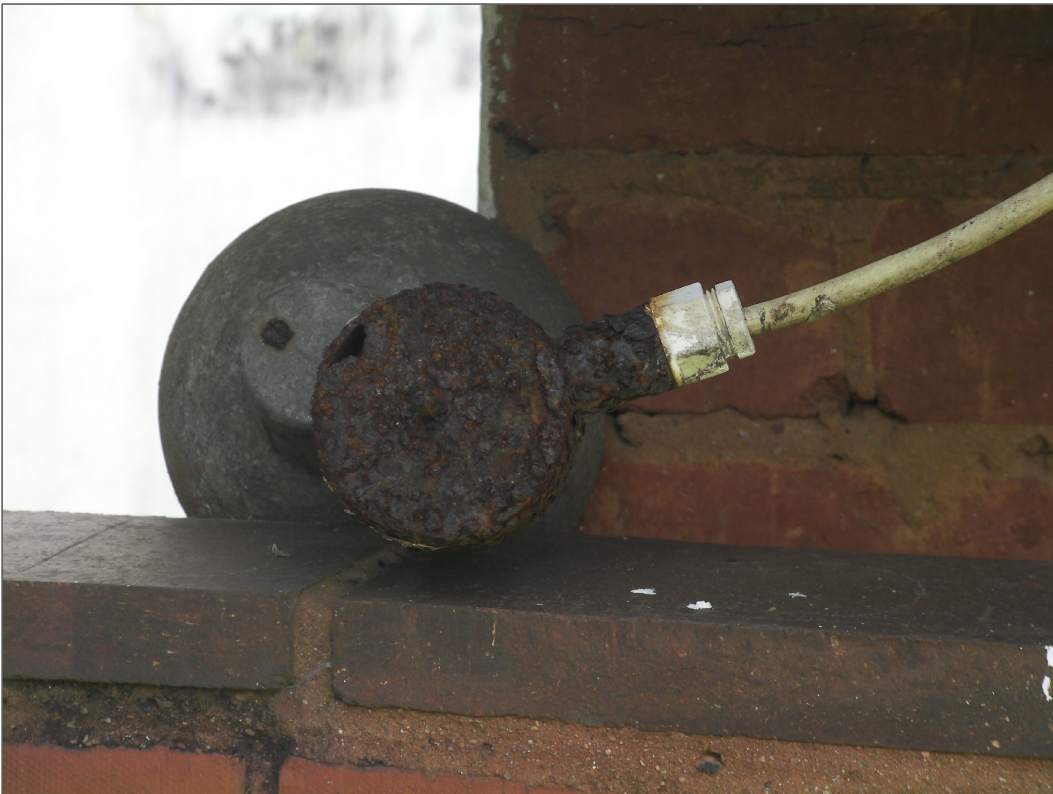
PHOTOGRAPH 20 -----VIEW OF LIGHT FITTING - HOUSING TO ELECTRICAL CONNECTION IS ALSO RUSTING AWAY - FITTING IS LYING LOOSE WITH SUB STANDARD CONNECTION (DANGEROUS)
