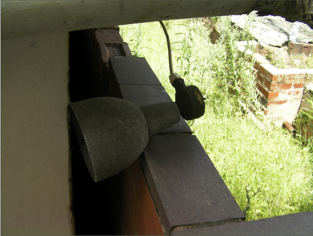
PHOTOGRAPH 19 -----VIEW OF LIGHT FITTING - HOUSING TO ELECTRICAL CONNECTION IS ALSO RUSTING AWAY - FITTING IS LYING LOOSE WITH SUB STANDARD CONNECTION (DANGEROUS)
