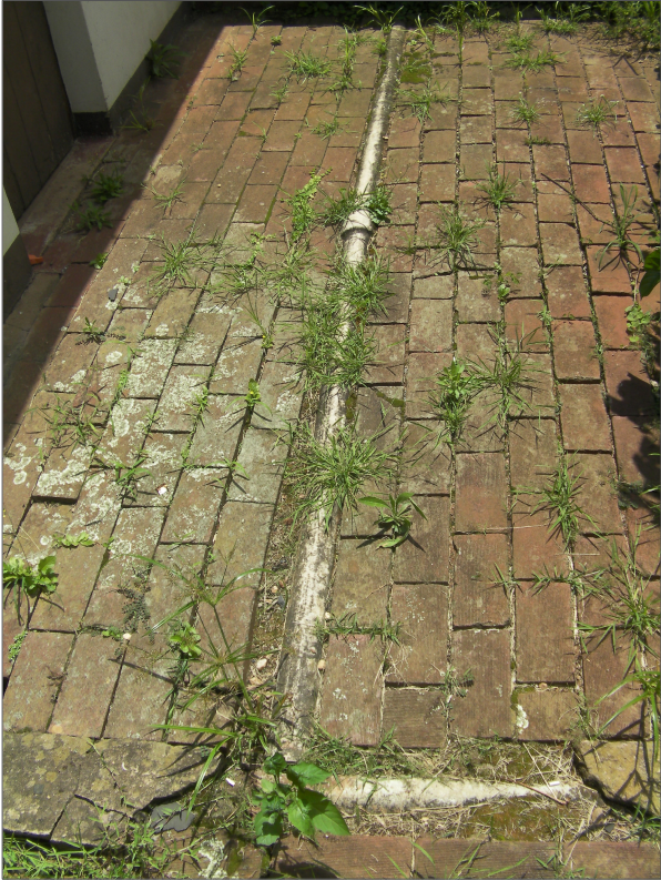
PHOTOGRAPH 21 ---- SEWER PIPE IS EXPOSED - LAID AT PAVING LEVEL WITH PIPE FALLING IN TWO DIFFERANT DIRECTIONS
