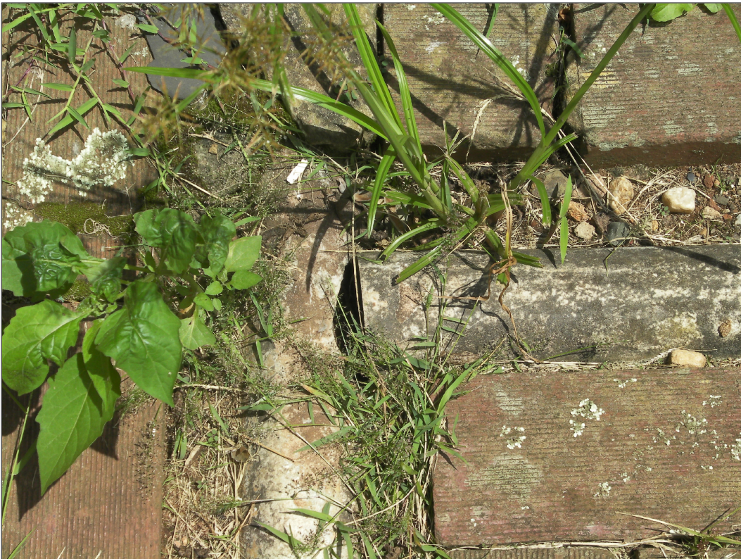
PHOTOGRAPH 22 ---- SEWER PIPE IS EXPOSED - CONNECTION BETWEEN TWO PIPES INCORRECT THERE IS A HUG GAP THAT WILL ALLOW FOR THE SEWER TO LEAK ONTO THE PAVING
