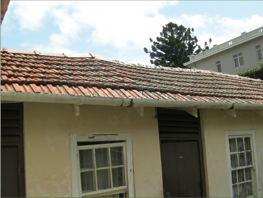
PHOTOGRAPH 23 ---- VIEW OF EXISTING MAIDS QUARTERS - ROOF STRUCTURE IS BORER INFESTED (ROOF TILES ARE BOWING)
