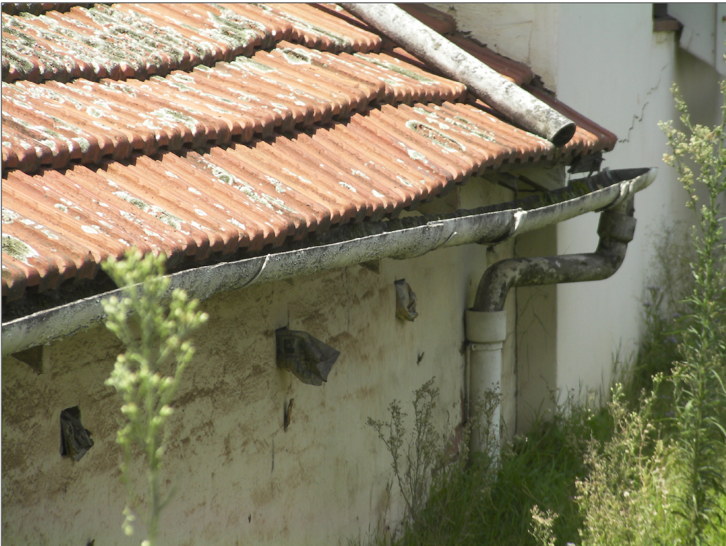
PHOTOGRAPH 24 ---- VIEW OF EXISTING MAIDS QUARTERS - ROOF STRUCTURE IS BORER INFESTED (ROOF TILES ARE BOWING & GUTTERS ARE FALLING OFF)
