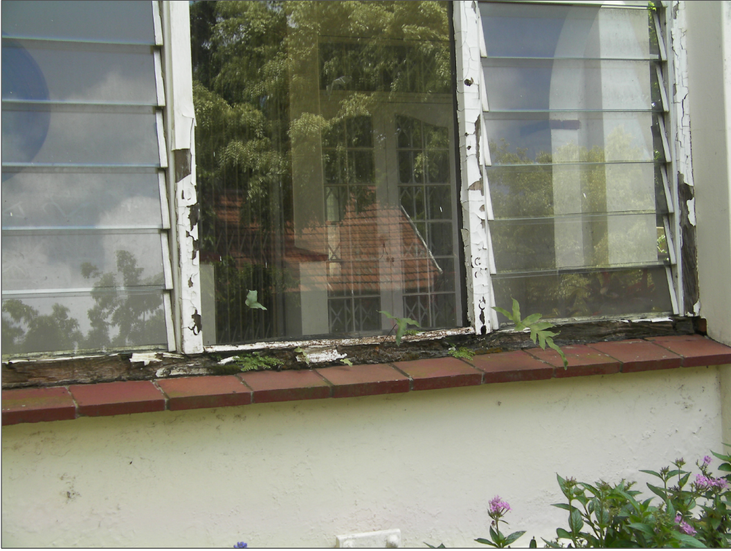
PHOTOGRAPH 25 ---- BORER INFESTED WINDOW FRAME
