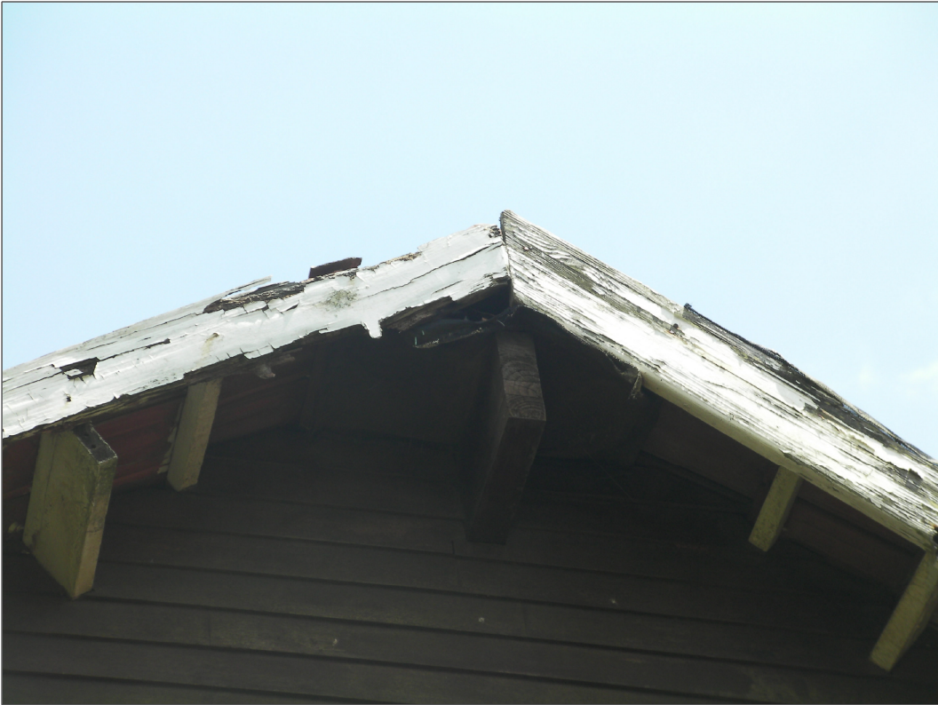
PHOTOGRAPH 26 ---- BORER INFESTED FASCIA BOARD
