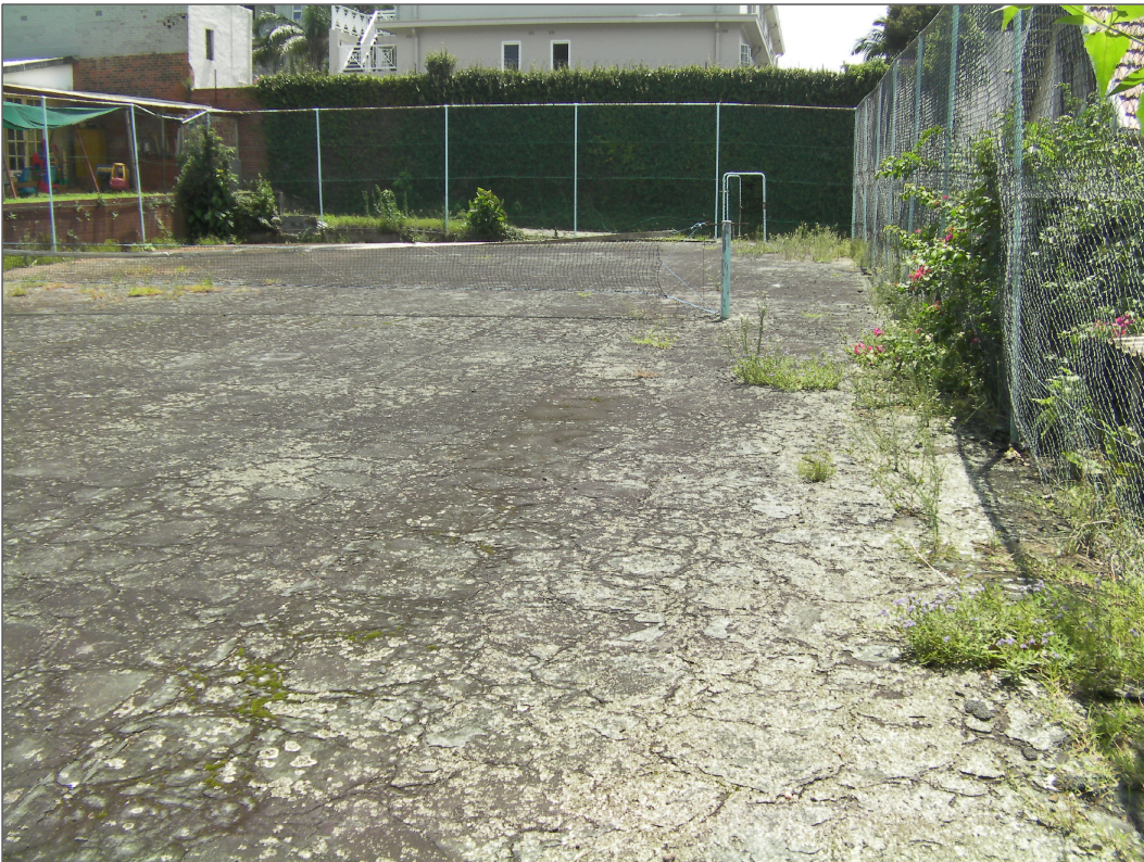
PHOTOGRAPH 28 ---- VIEW OF EXISTING TENNIS COURT IN A DILAPIDATED STATE
