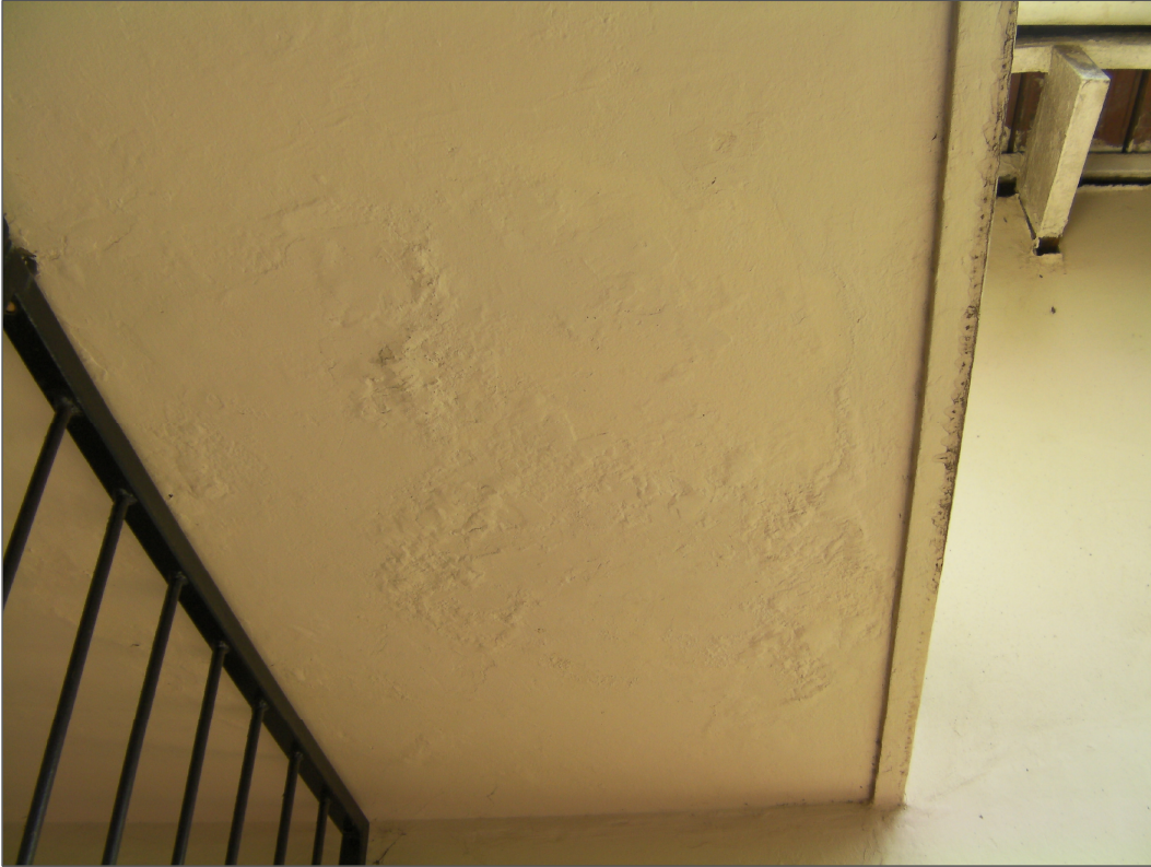
PHOTOGRAPH 27 ---- EXISTING CONCRETE ROOF SLAB HAS DAMPNESS PROBLEMS
