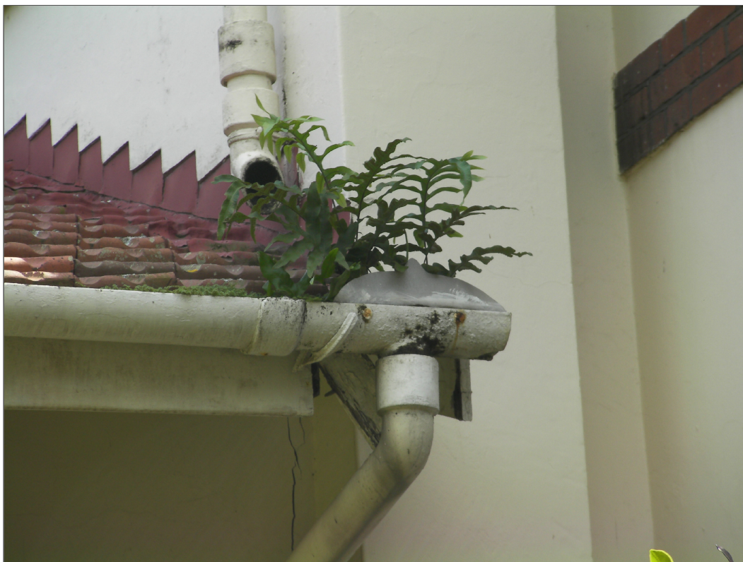
PHOTOGRAPH 29 ---- LACK OF MAINTENANCE IS EVIDENT IN THIS PHOTO
