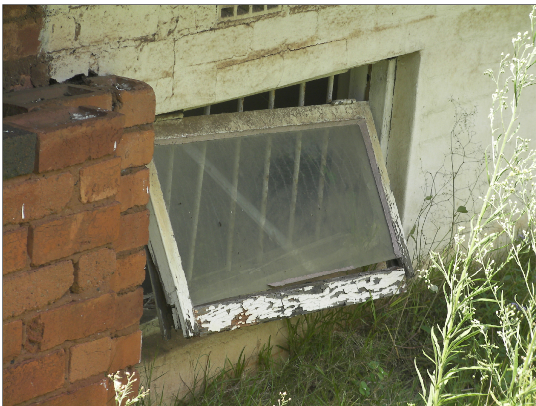
PHOTOGRAPH 30 ---- BORER INFESTED WINDOW IS SUPPORTED BY ONE HINGE
