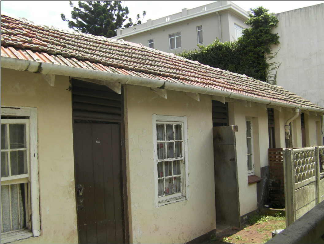
PHOTOGRAPH 4 ---- VIEW OF EXISTING MAIDS QUARTERS OUTBUILDING IS IN A POOR CONDITION - BORER INFESTED
