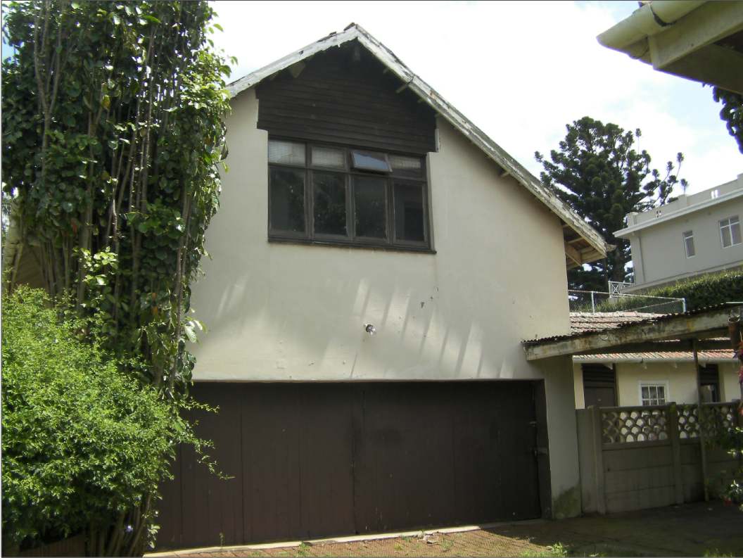
PHOTOGRAPH 5 ----- VIEW OF EXISTING GARAGE BUILDING WITH ROOM ABOVE FASCIA BOARDS ARE FALLING OFF IN SOME PLACES
