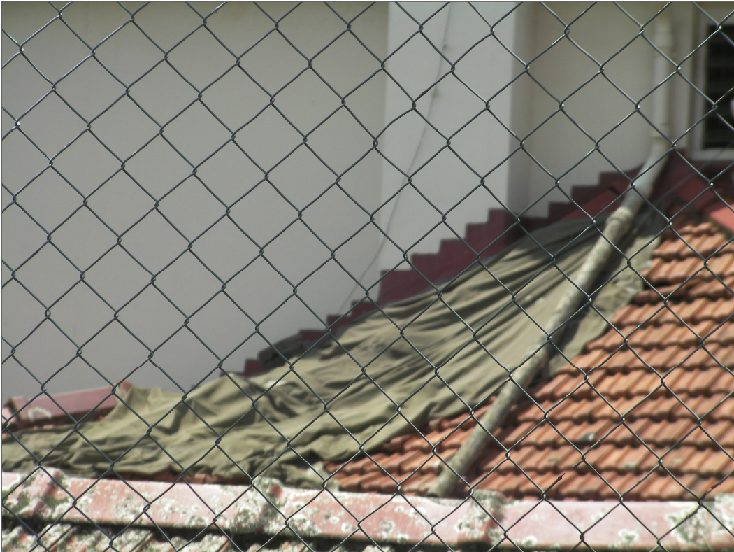
PHOTOGRAPH 16 ----- VIEW OF PART OF THE ROOF THAT HAS COLLAPSED - AREA IS COVERED WITH SOME SORT OF MATERIAL - ENTIRE ROOF IS BORER INFESTED
