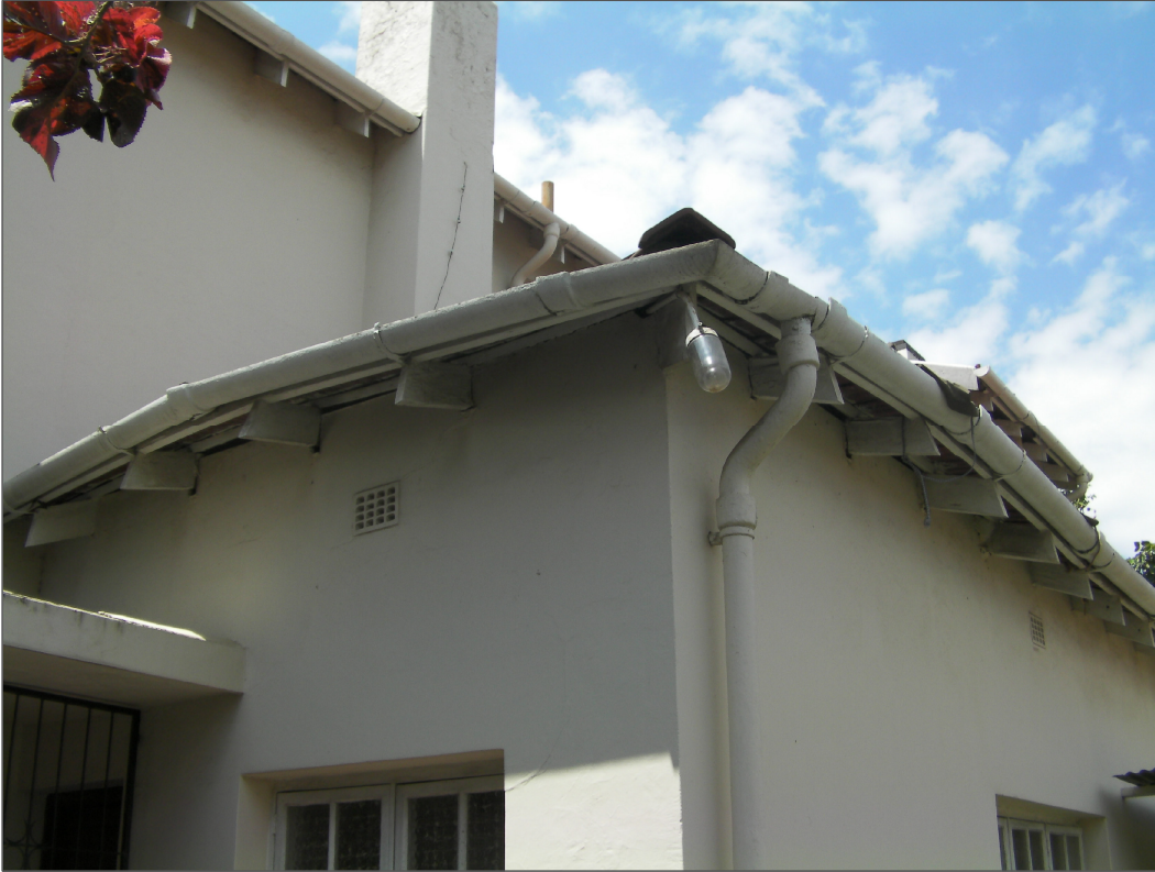
PHOTOGRAPH 15 ----- VIEW OF EXISTING ROOF THAT HAS FALLEN IN (REFER TO PHOTO BELOW FOR TOP VIEW)
