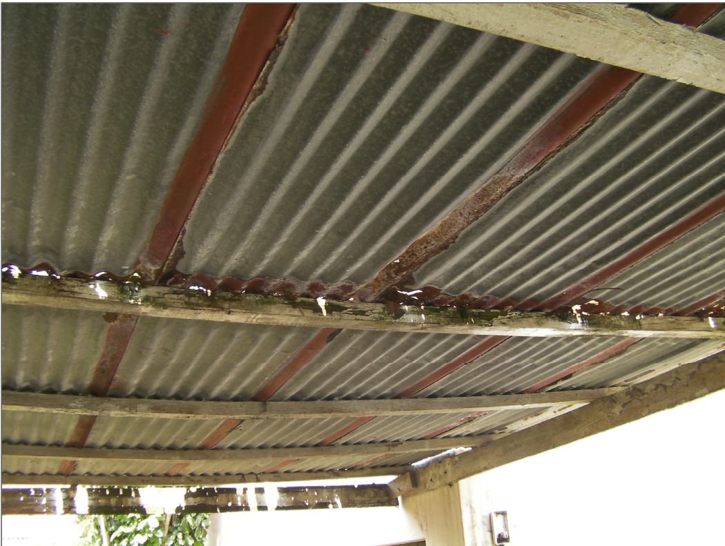
PHOTOGRAPH 18 ---- VIEW OF CARPORT - THIS STRUCTURE IS ABOUT TO COLLAPSE ROOF SHEETING HAS ALMOST RUSTED AWAY
