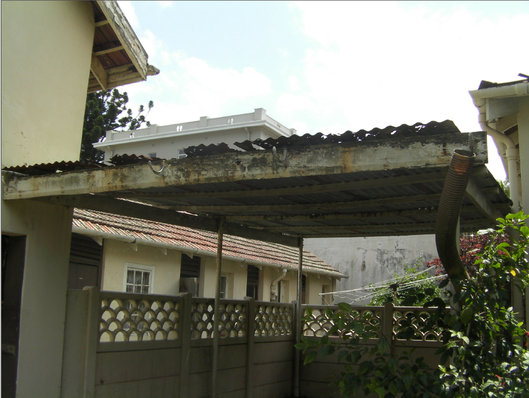
PHOTOGRAPH 17 ---- VIEW OF CARPORT - THIS STRUCTURE IS ABOUT TO COLLAPSE ROOF SHEETING HAS ALMOST RUSTED AWAY
