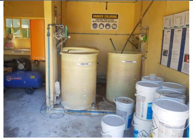
Thorndale Dam WTW Chemical dosing
