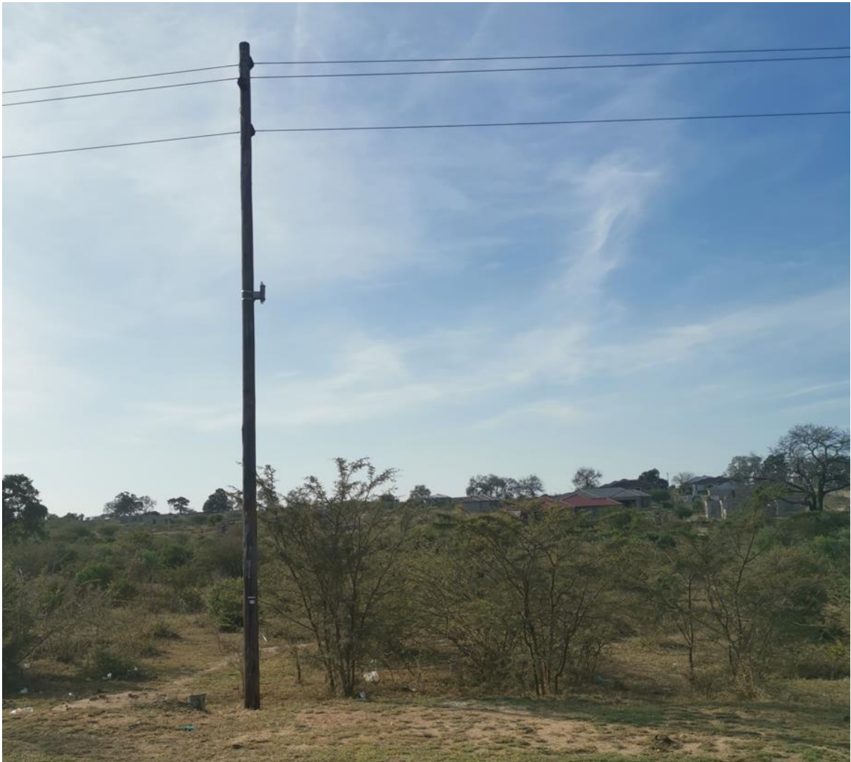
Figure 17 Electrical lines in vicinity of site
