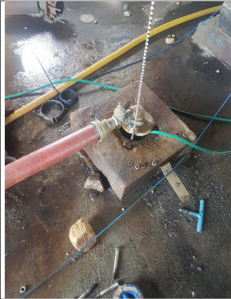
Thorndale Dam pumping main held up by rope to avoid sucking up Debre
