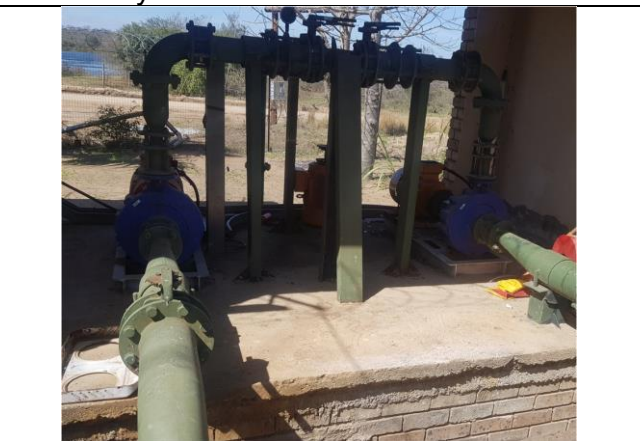
Thorndale Dam WTW Pumping Main Pump Station
