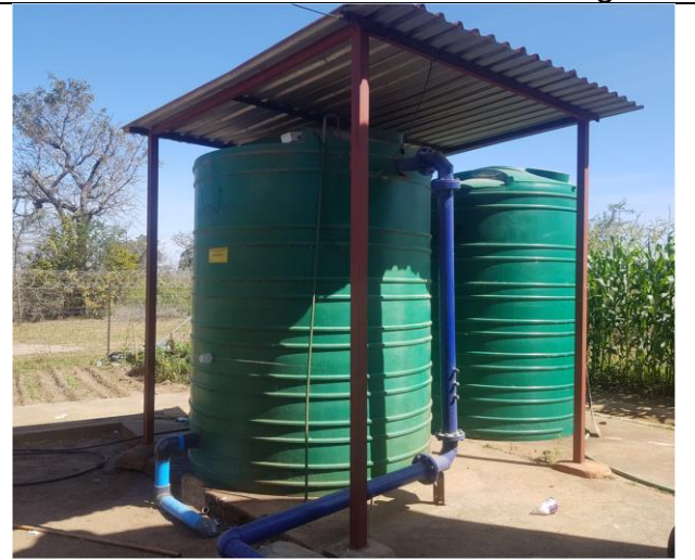
Potable water storage tank. One connected and one yet to be connected
