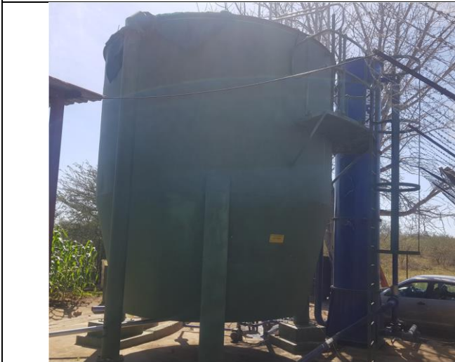
Thorndale Dam WTW dosing tank and settling tank
