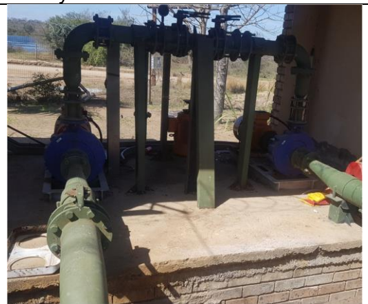
Thorn Dam WTW Pumping Main Pump Station
