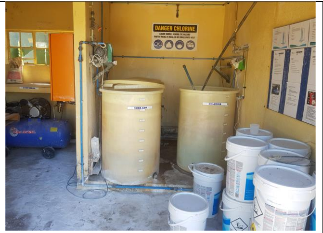
Thorn Dam WTW Chemical dosing
