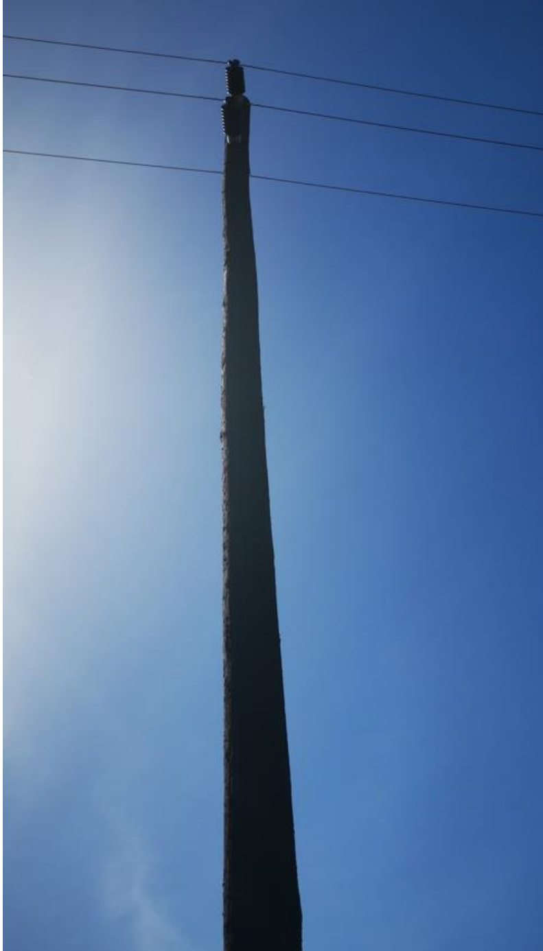
Figure 16 Electrical lines onsite
