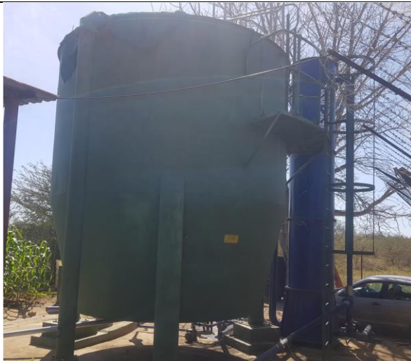
Thorn Dam WTW dosing tank and settling tank
