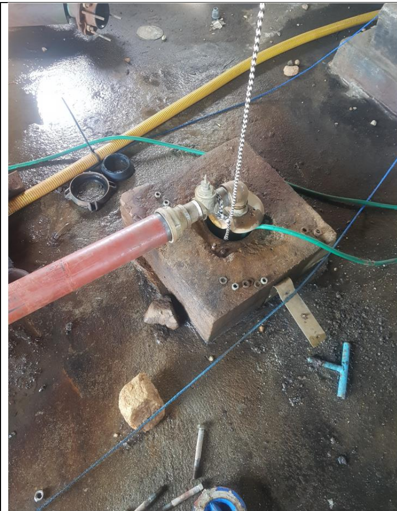
Thorn Dam pumping main held up by rope to avoid sucking up Debre
