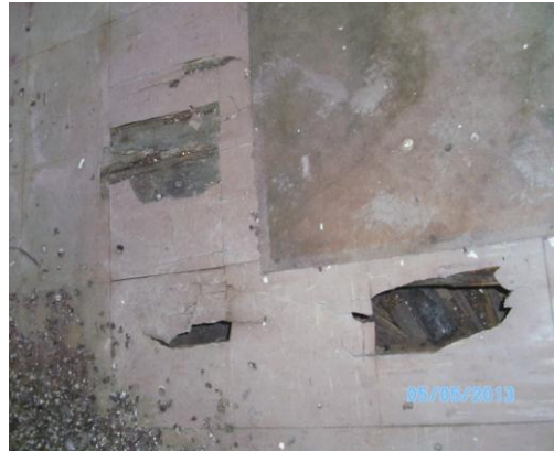
Tiles floor with holes and bird droppings
