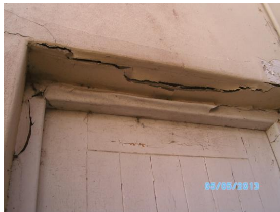
Structural failure on the door
