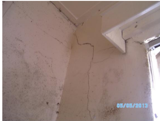
Crack on the wall inside
