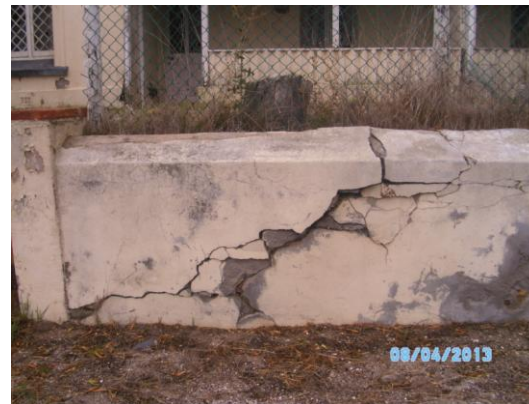
Fence wall has cracks caused by traffic vibration
