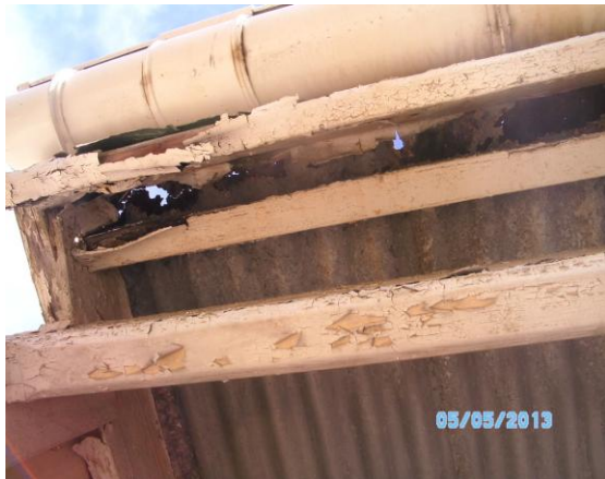
Rusting Corrugated iron sheets
