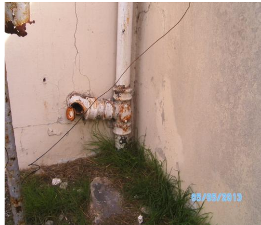
rusting of drainage pipe
