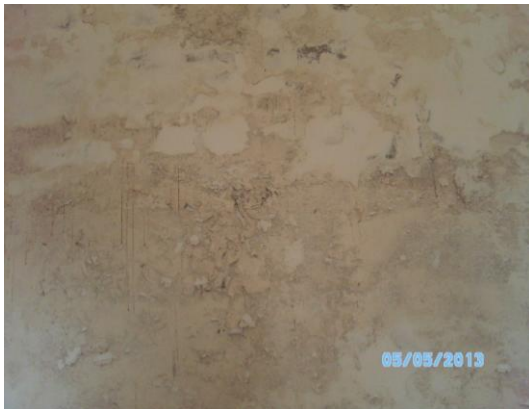
Condition of the plaster in side (Crumble)
