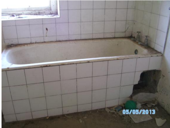
Condition of the showed basin
