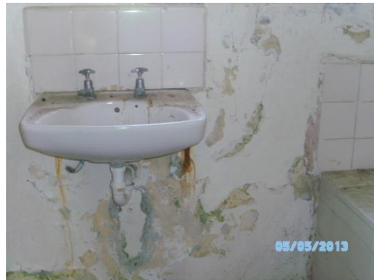
Effect of moisture on the wall
