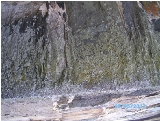
Fungus on the Southern wall (un plastered)
