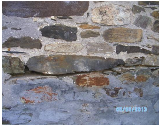
Mortar detached on un plastered wall
