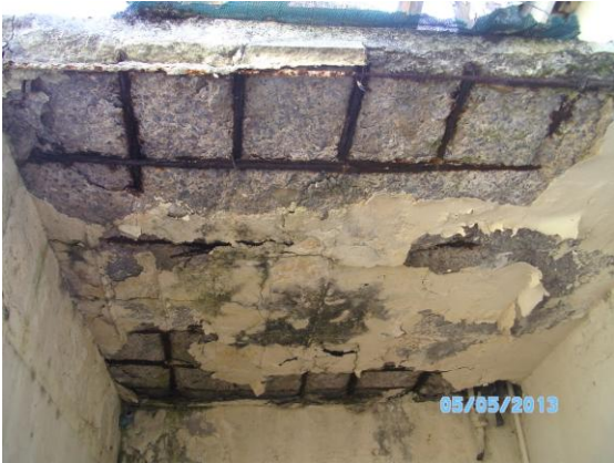
Corrosion of Reinforcement on the slab
