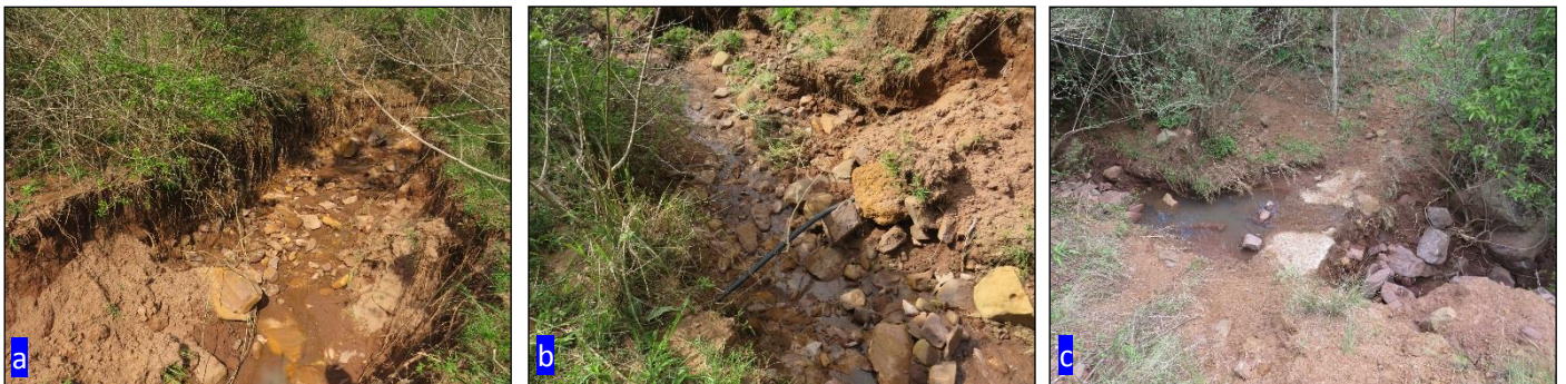
Figure 18: (a): Incised watercourse channel at WC34; (b): Image of the exposed waterpipe within the drainage channel at WC34; (c): Existing pipeline encased in concrete at WC35.
