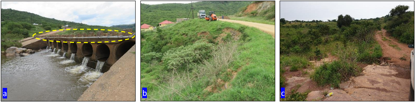
Figure 16: (a): The pipeline tied onto the bridge structure at WC42 is in poor condition and requires replacement; (b): The pipeline route follows the existing gravel road at WC47; (c): Exposed bedrock visible at WC51.
