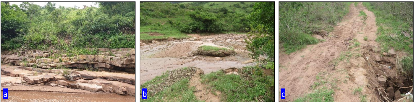
Figure 17: (a): The watercourse at WC57 is flanked by a wall of rock; (b): Water course and CVB wetland to be crossed by water pipeline at WC59; (c): Gravel road showing signs of erosion at WC33.
