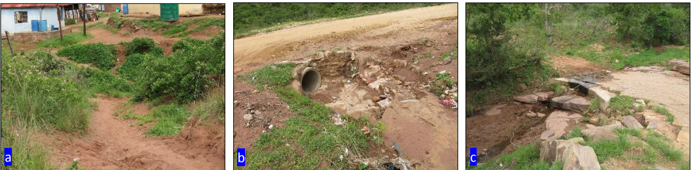
Figure 14: (a): Pipeline to cross at WC31 to provide a yard connection for these households; (b): Pipeline to cross at WC32 along an existing gravel road; (c): Existing pipeline encased in concrete at WC36.
