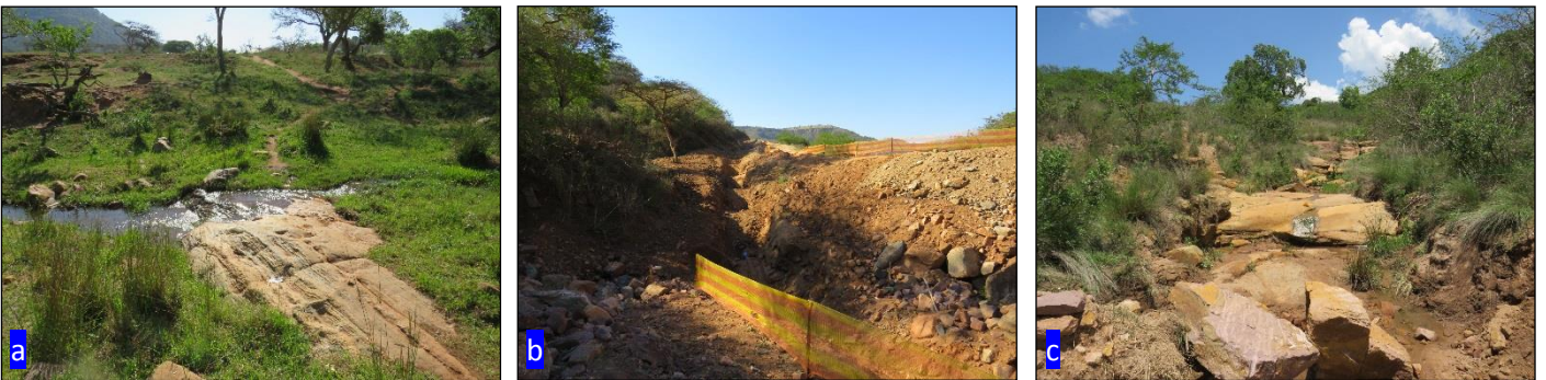
Figure 13: (a): Small drainage line located at WC 21. The pipeline will follow an existing footpath and the existing pipeline route; (b): Phase 2 of the uMshwathi WSS currently taking place. The smaller reticulation pipeline will follow the same route as the bulk pipeline currently being installed (WC23); (c): Rocky terrain and drainage lines noted throughout.
