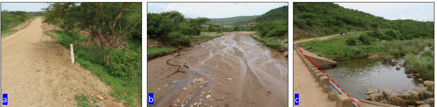
Figure 15: (a): Existing pipeline noted at WC37. (b): The pipeline crossed the channelled valley bottom wetland leading into the Mvoti River at WC38; (c): Bridge with existing pipeline tied to the structure over the Mvoti River (WC42).
