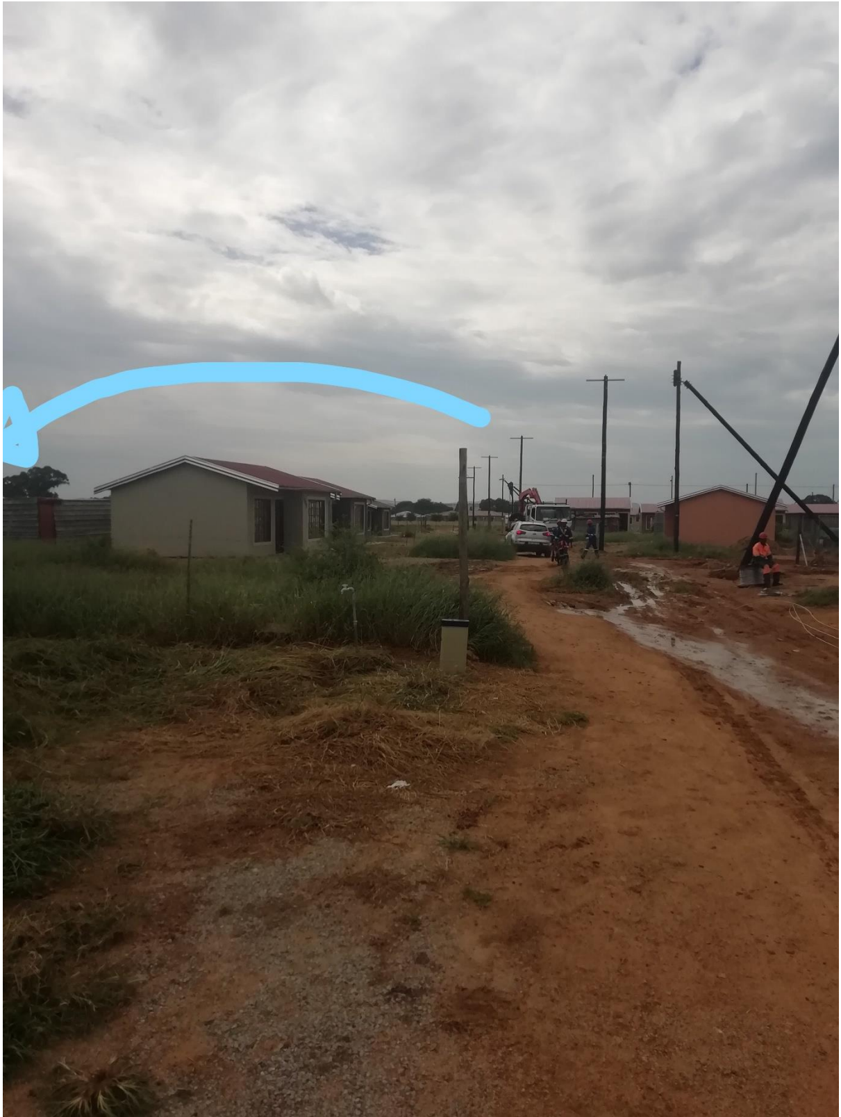
3.3 The new line under construction street front, the blue line points to where the graveyard is behind the houses
