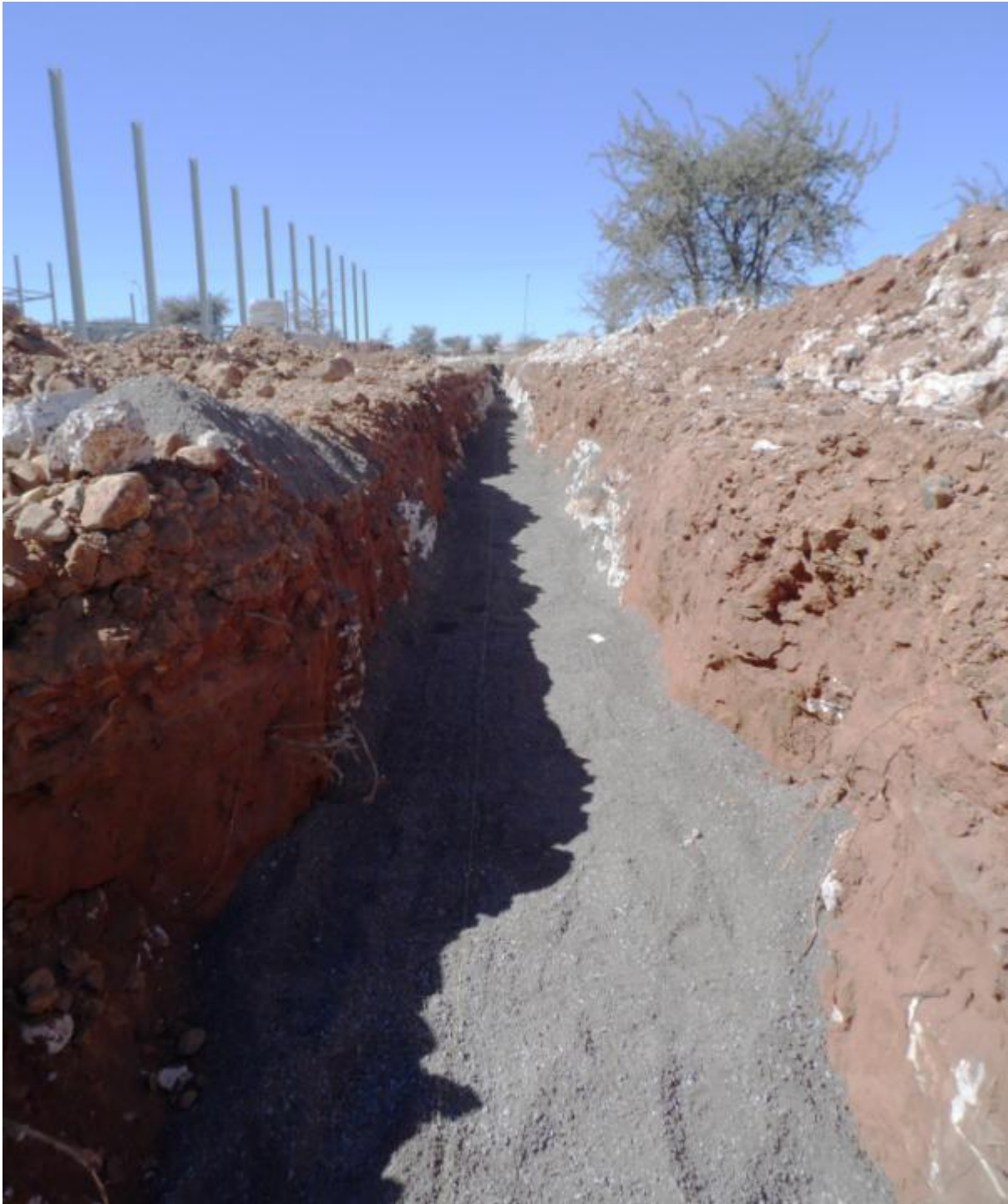
Figure 36: Developer trench from the western end looking east (deposit is mostly sand, with some calcrete)
