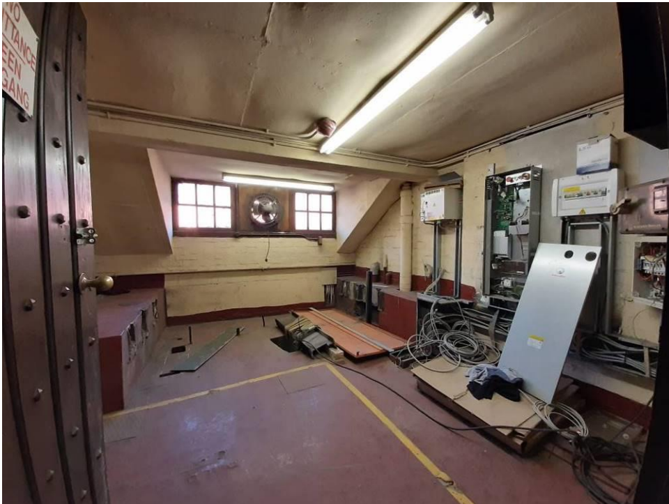
Fig. 83_Lift room located in the East wing above the Goods Lift shaft (Source: tsica heritage consultants, 09.07.2019)
