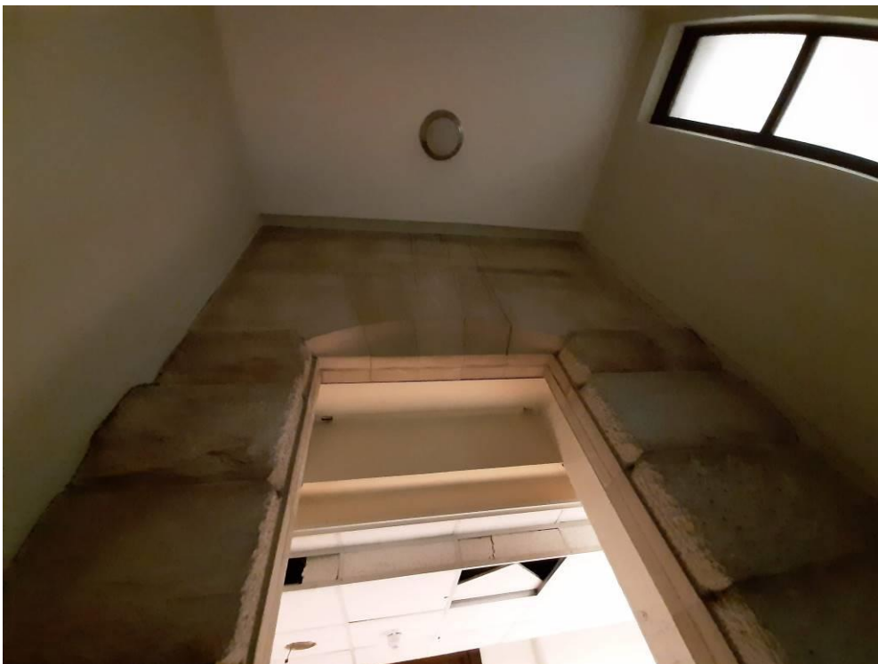
Fig. 41_Presidential Lift_original façade along the western elevation is untouched (Source: tsica heritage consultants, 09.07.2019)
