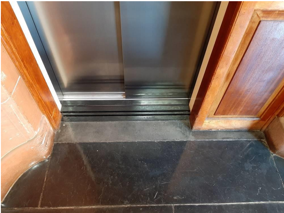
Fig. 52_Detail of floor landing interface of Passenger lift, all stone work and wooden cladding was put back in place and not damaged after lift was replaced (Source: tsica heritage consultants, 09.07.2019)
