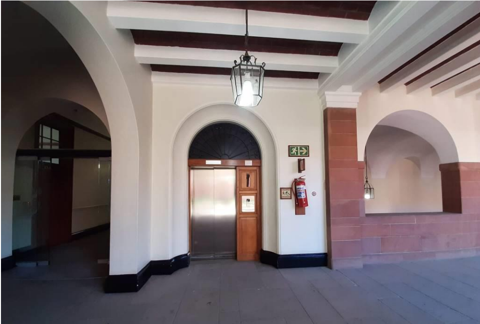
Fig. 73_Passenger lift for the public replaced along the southern side of the main staircase (Source: tsica heritage consultants, 09.07.2019)
