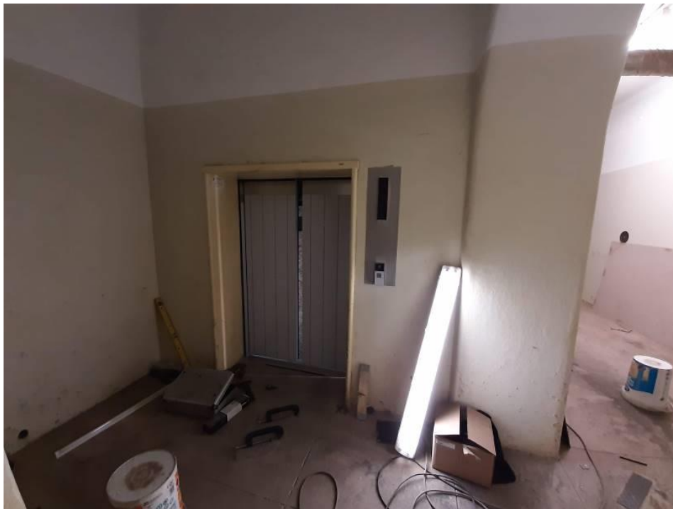
Fig. 26_Goods Delivery Lift replaced and work still in progress (Source: tsica heritage consultants, 09.07.2019)
