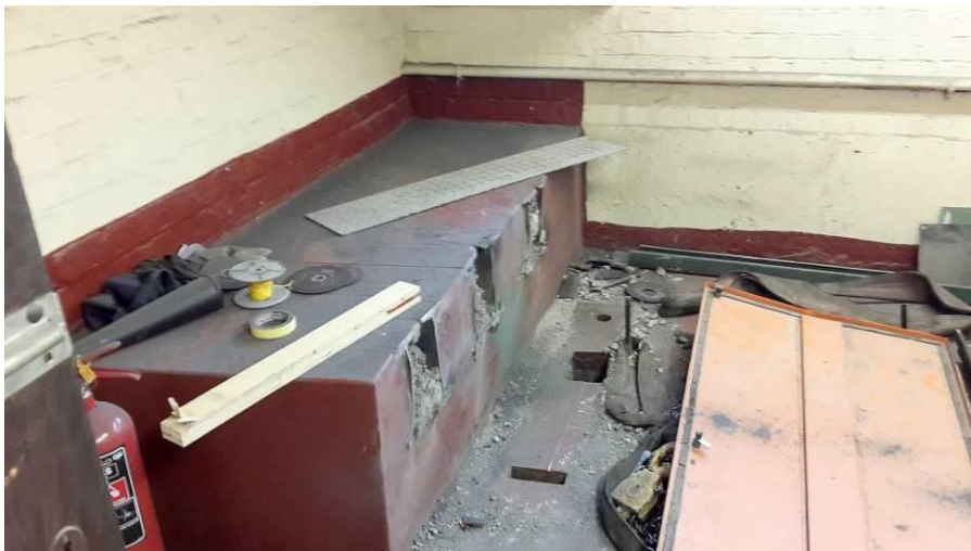
Fig. 87_ Lift room located in the East wing during the construction phase (Source: tsica heritage consultants, 09.07.2019)
