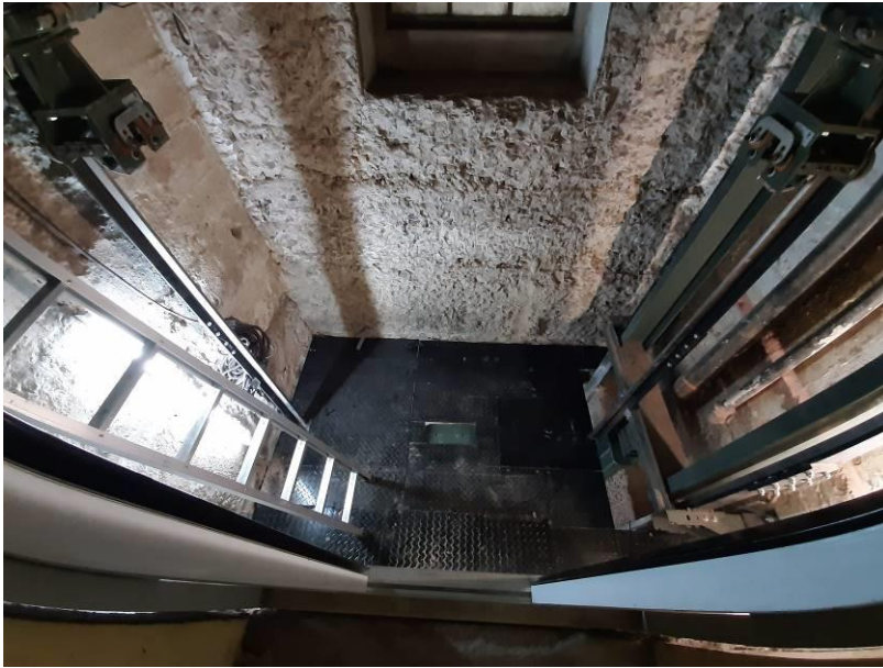
Fig. 27_ Goods Delivery Lift replaced and water issue resolved (Source: tsica heritage consultants, 09.07.2019)
