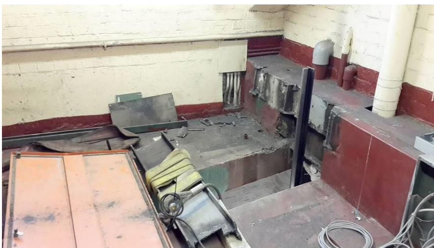
Fig. 88_ Lift room located in the East wing during the construction phase (Source: tsica heritage consultants, 09.07.2019)
