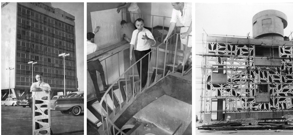
Insert 7a. Warunkiewicz on site, directing the installation of artworks. Right, the stunning screen of the south access tower. (photo credits: Marek Warunkiewicz via Facts about Durban)
