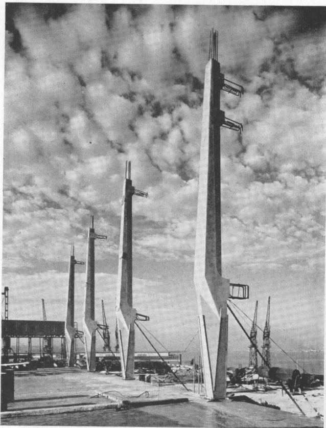
Carefully designed precast concrete columns being erected to support the main concourse.
