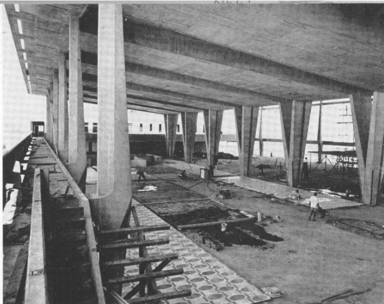
Main concourse under construction showing precast columns in position and terrazzo floor slabs being laid.
