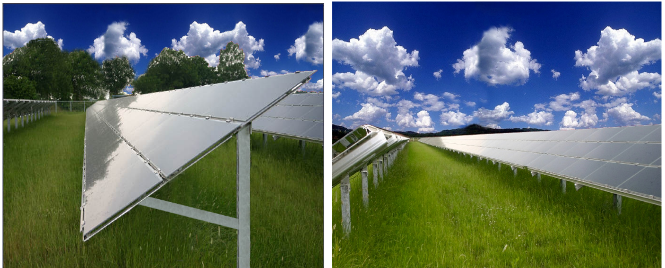
Figure 4: Lateral views of PV arrays mounted on fixed mounting systems
