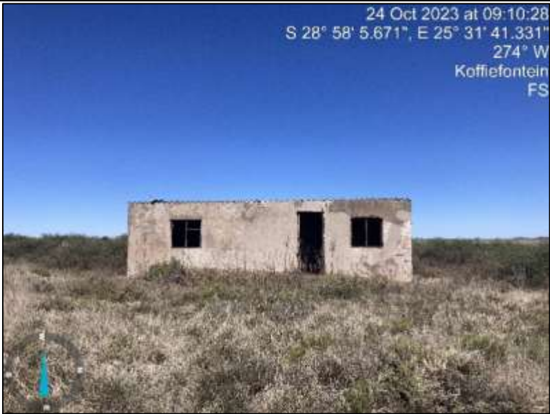
Figure 48: A ruin farm worker house.
