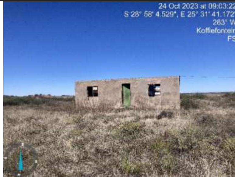
Figure 44: A ruin farm worker house.
