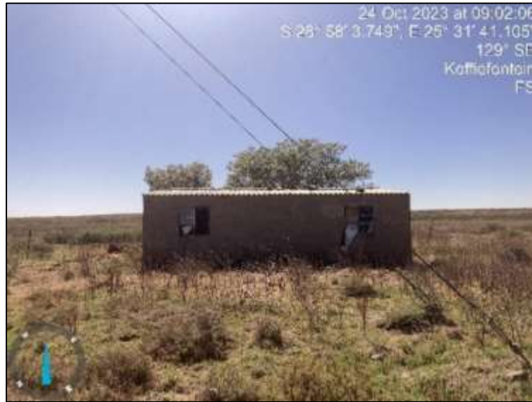
Figure 42: A ruin farm worker house.
