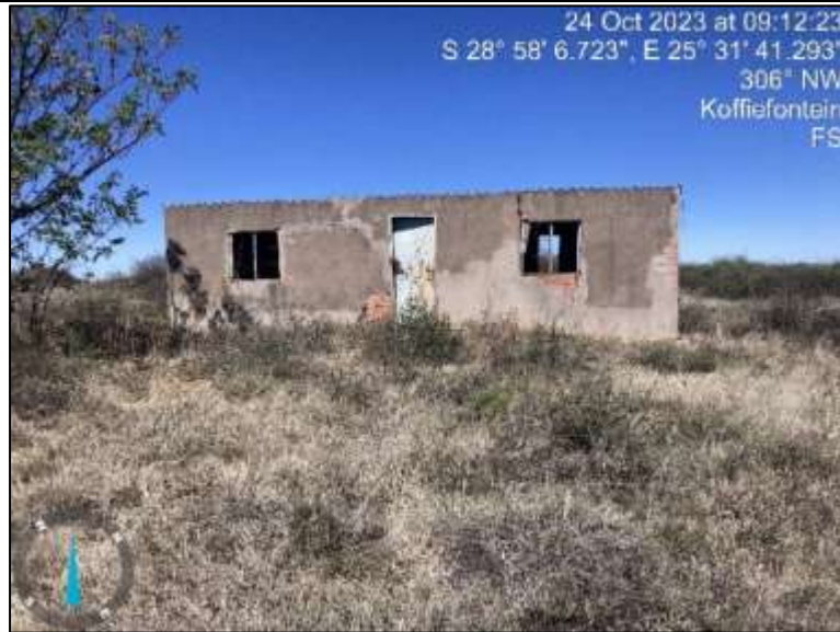
Figure 46: A ruin farm worker house.
