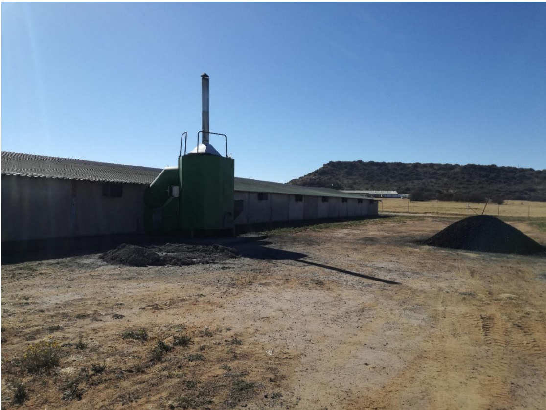
Figure 6 – Hot air system for heating of the breeders houses.
