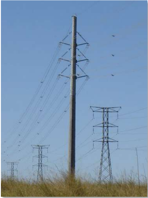
Figure 4-7: Example of a Self-supporting Monopole (foreground) and Lattice Structure (background)
