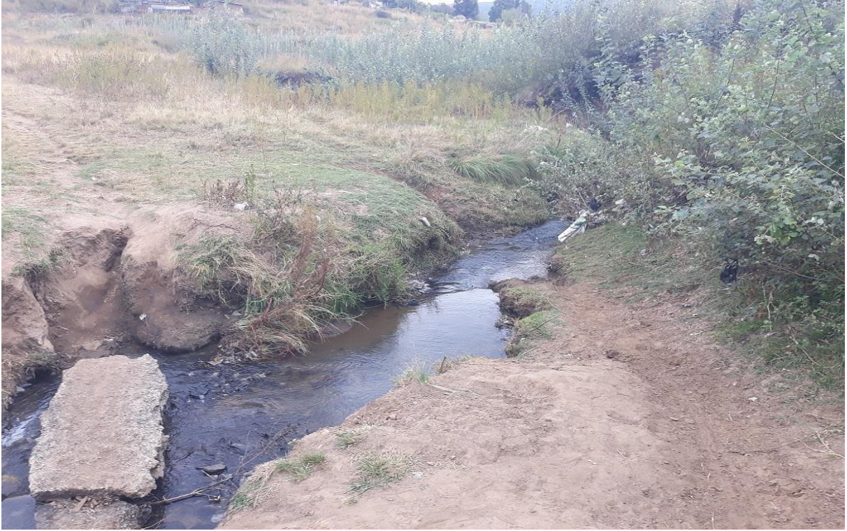
FIGURE 20: REMNANTS OF SMALL FOOTBRIDGE AT THE PHOPHOPHO VILLAGE BRIDGE SITE.
