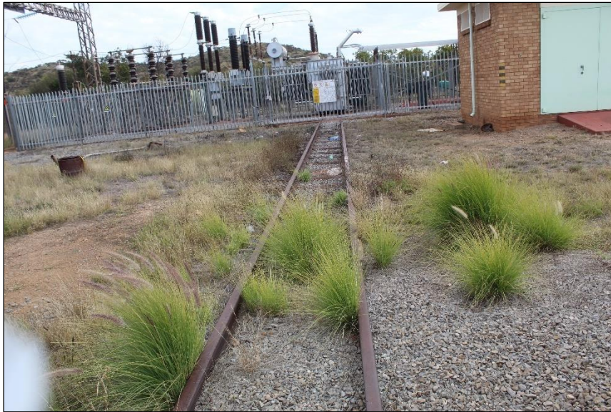
Figure 10: The electrical substation seen from the east. It was built at the terminal of a short railway line. The main line is behind the camera running parallel with the perimeter fencing of the substation in front of the camera.
