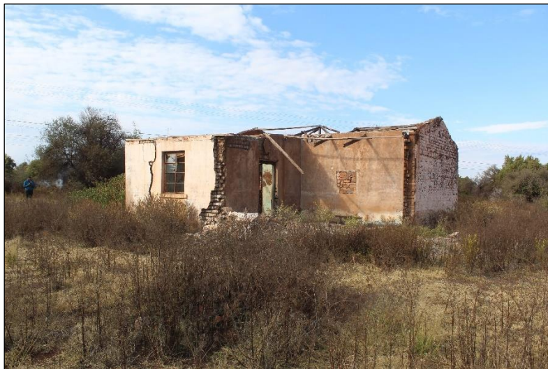
Figure 2: View of the east and north elevation of the building shows a room with two walls which have collapsed
