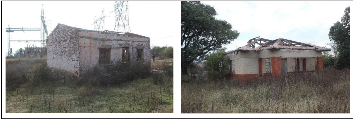
Figure 12: The two service buildings at the Palingspan railway siding. Left – the building under study; Right – the main building situated north of the substation.
