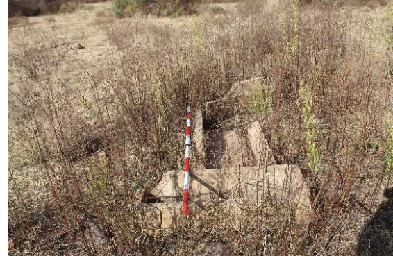
Figure 15: Broken concrete used for watering livestock
