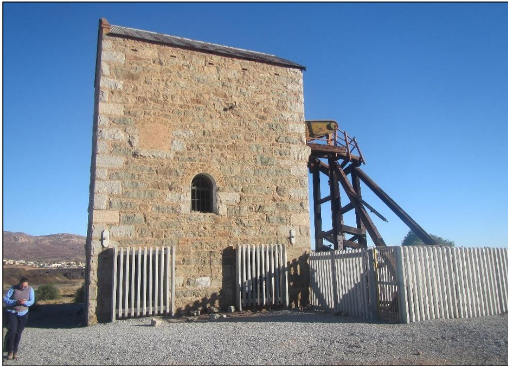
Figure 43: View of the east face of the Cornish Beam Pump with its collapsing wooden scaffold.
