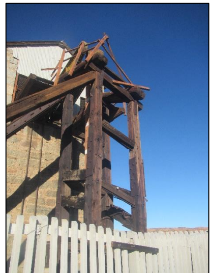
Figure 46: View of the Cornish Beam Pump wooden scaffold showing the partial collapse of the structure.
