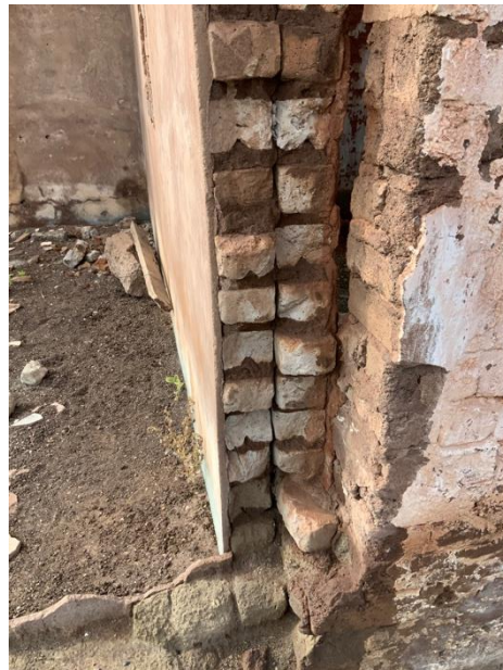
Figure 8. Detail of the brickwork junction between the original section and added section
