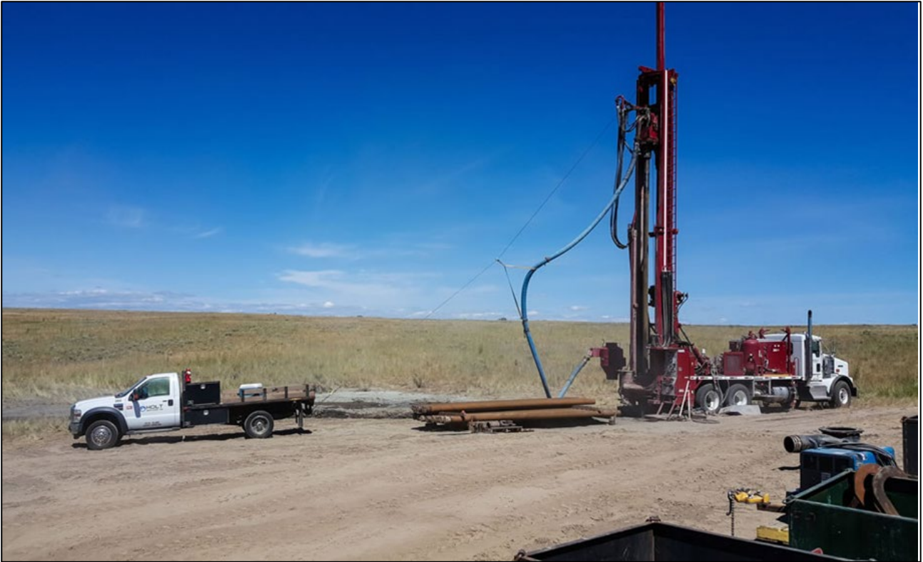
Figure 3: Example of a truck-mounted drill rig similar to that which would be used for this project.
