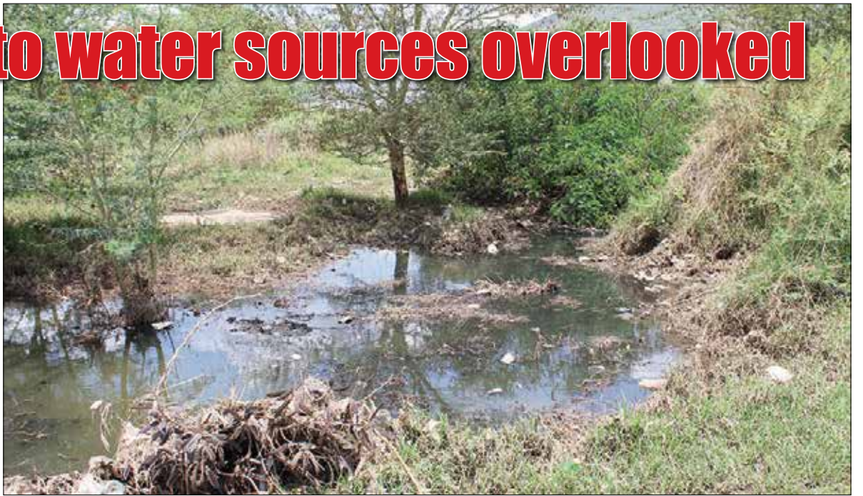
One of the disabled and unattended raw sewerage plants systems flowing into water sources in Sekhukhune district which carries a potential health risk to communities.
