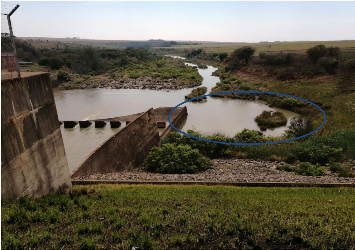
Photo Plate 5: The section which requires rehabilitation after erosion
