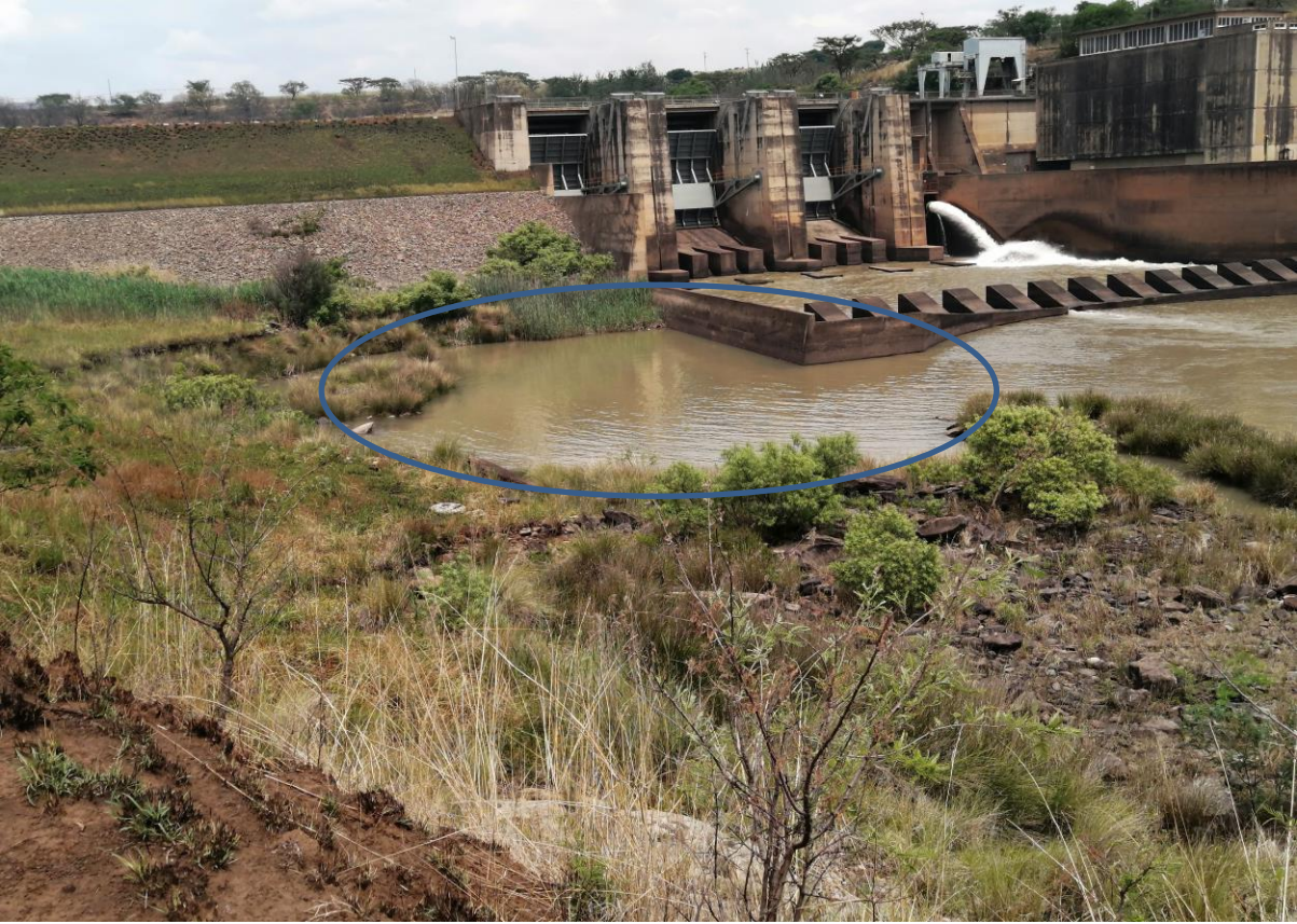
Photo Plate 7: The section which requires rehabilitation after erosion
