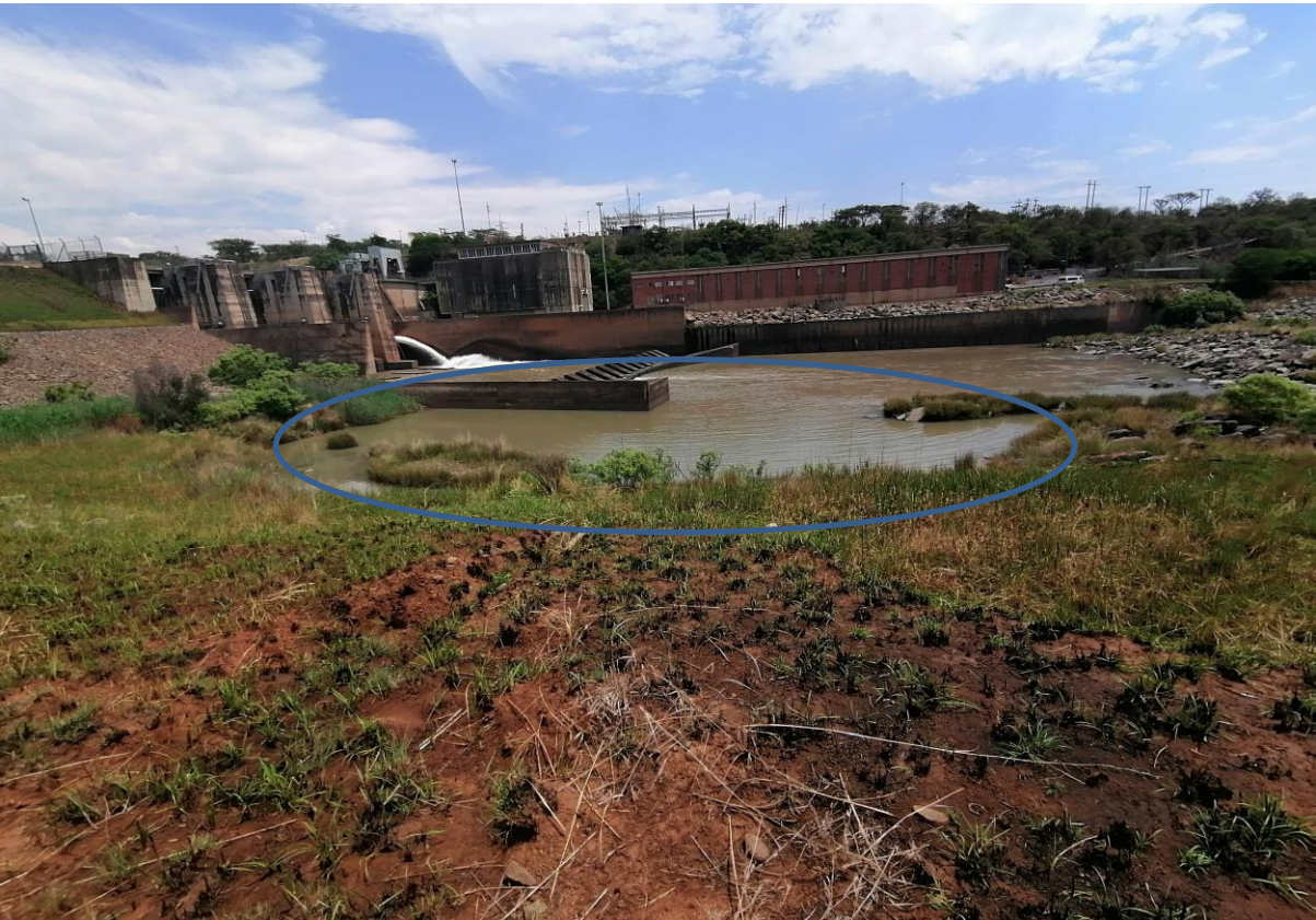
Photo Plate 8: The section which requires rehabilitation after erosion
