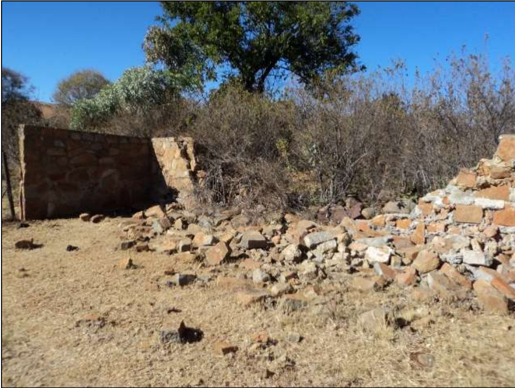
Figure 36: Dilapidated structure H04.
