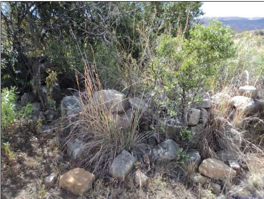
Figure 43: Dilapidated angular stone-wall enclosure H23.
