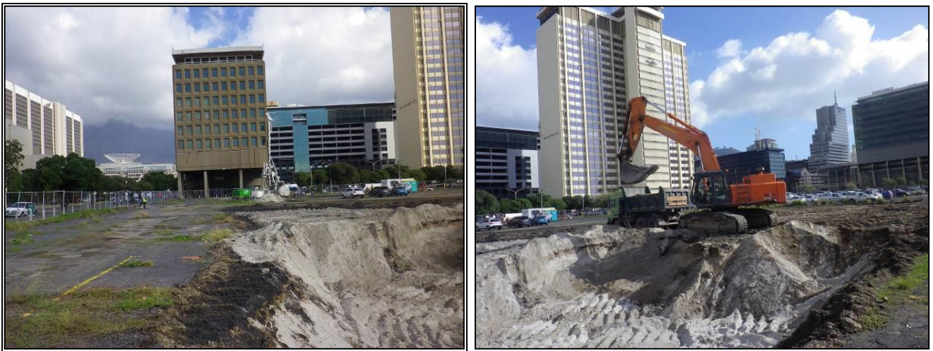
Plates 25 and 26: Bulk earthworks at Erf 247 in progress. A number of key buildings provide reference points. The uniform nature of the sub-surface deposits is clearly visible
