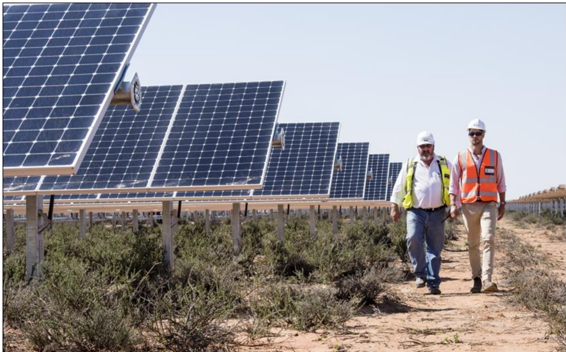
Figure 2: Photovoltaic (PV) solar panels. (Photo: SunPower Solar Power Plant – Prieska).
