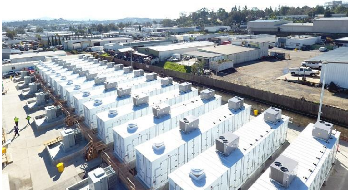
Figure 4: Aerial view of a BESS facility
