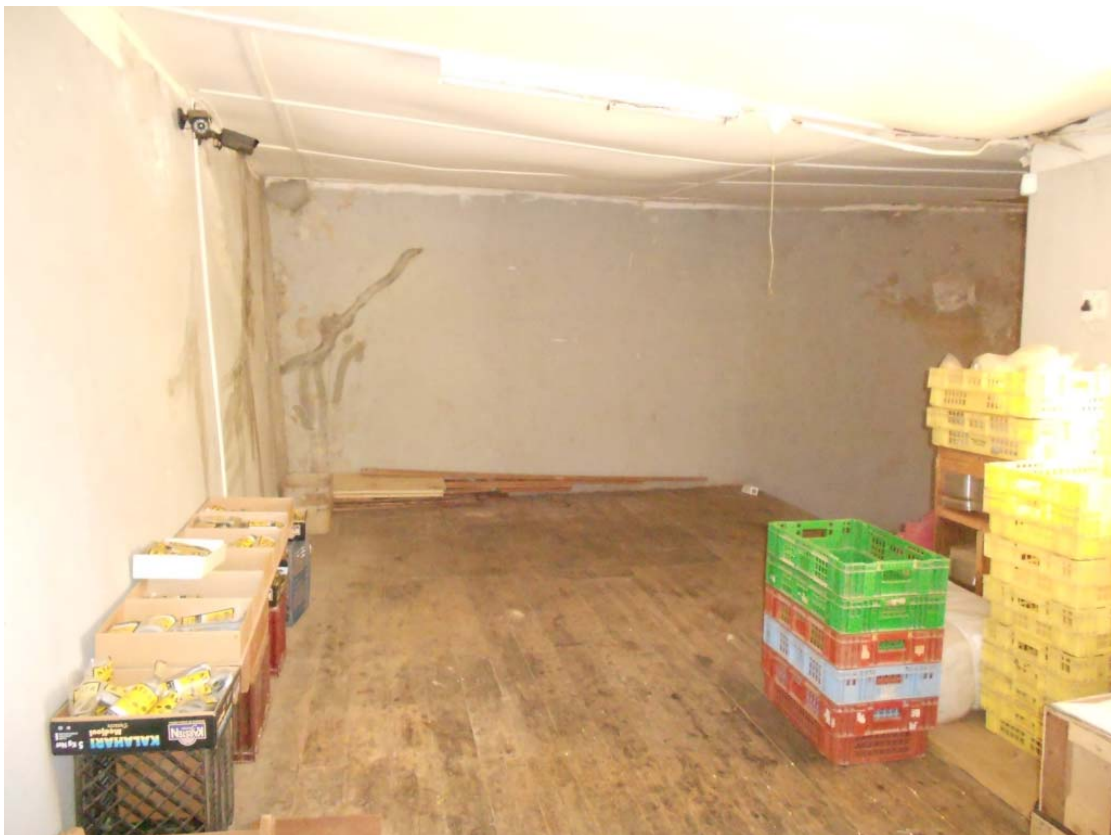
Photo 22: View inside upper level storeroom behind Atlas Trading looking towards existing hotel. Left-hand wall backs onto Danny's Auto.
