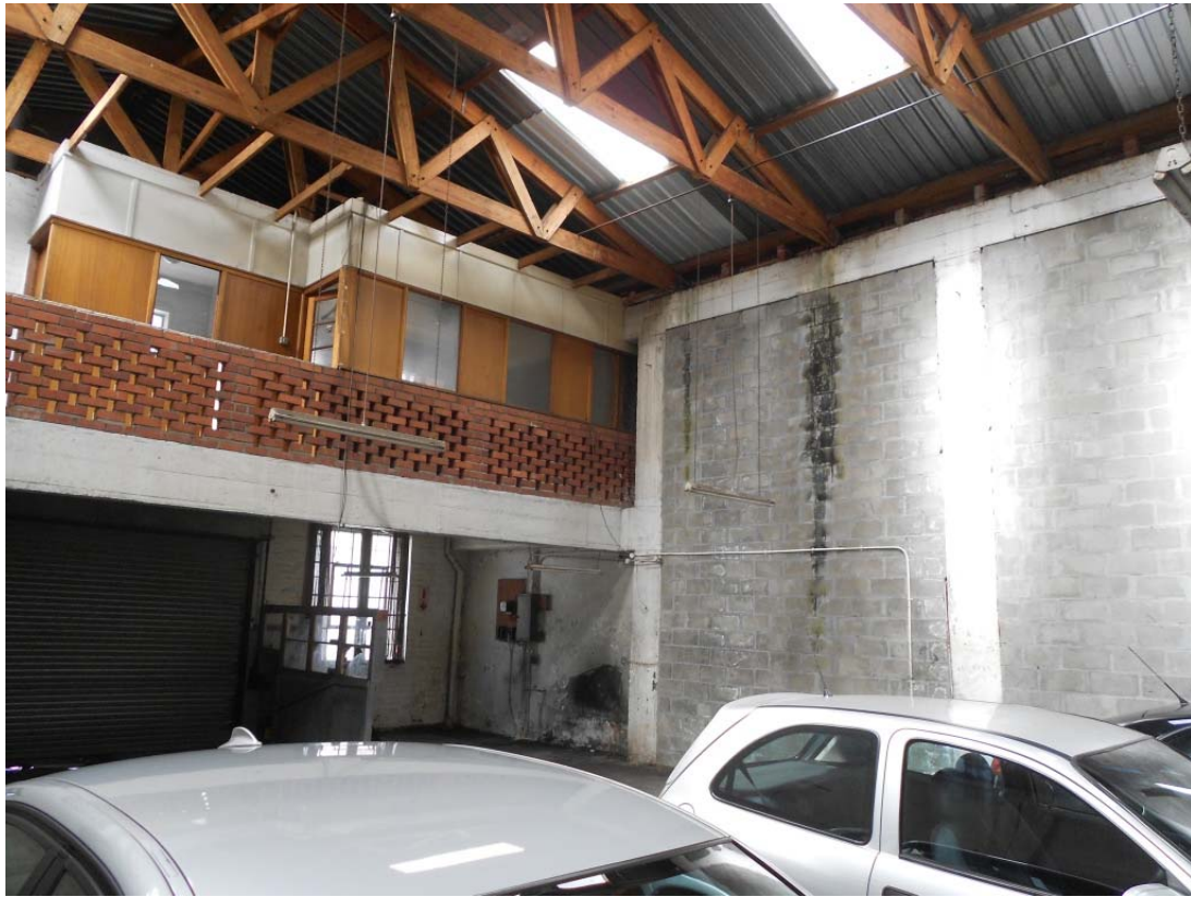
Photo 3: Internal view of Danny's Auto, showing contemporary concrete frame with brick infill panels.
