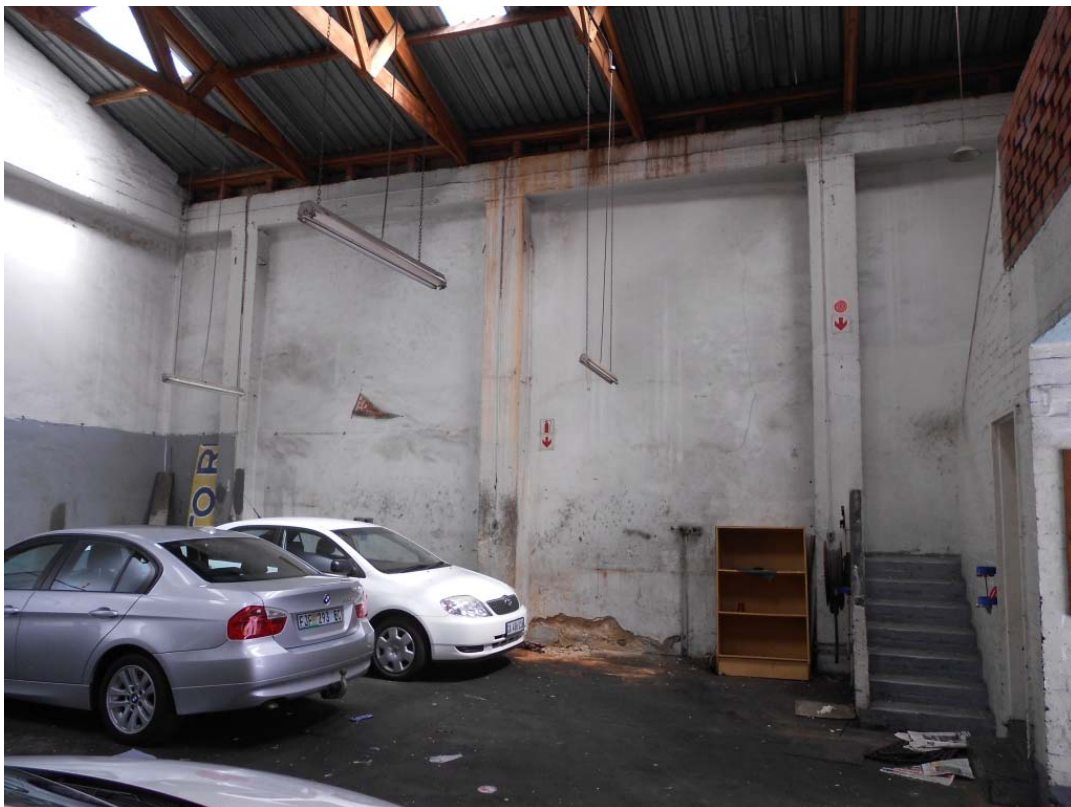
Photo 6: Internal wall of Danny's Auto being supported laterally by the concrete frame.
