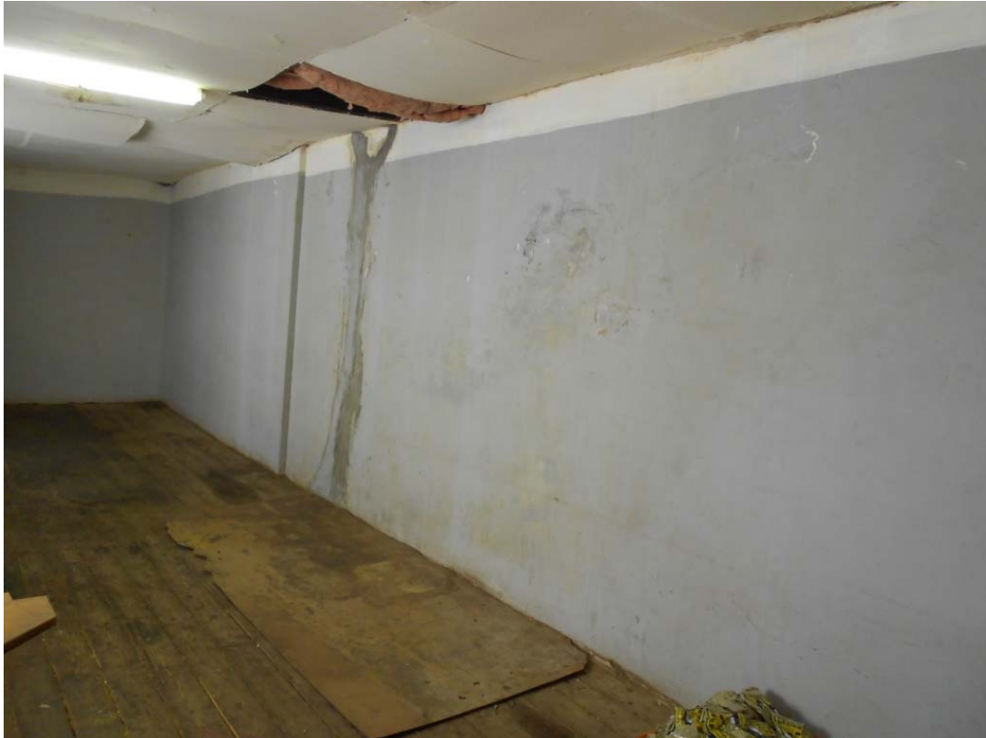
Photo 21: View inside upper level storeroom behind Atlas Trading. Right-hand wall backs onto Danny's Auto
