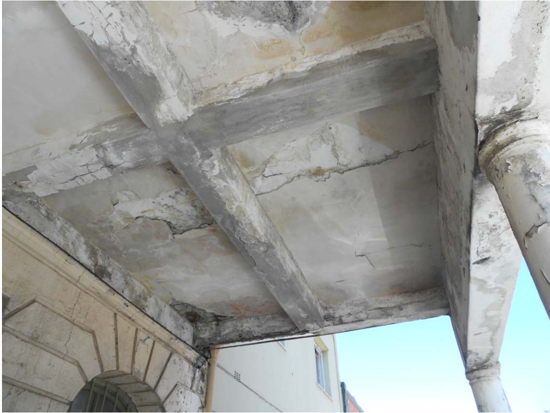
Photo 11: Balcony slab over the butchery entrance in Rose Street. Significant spalling and corroded reinforcement.
