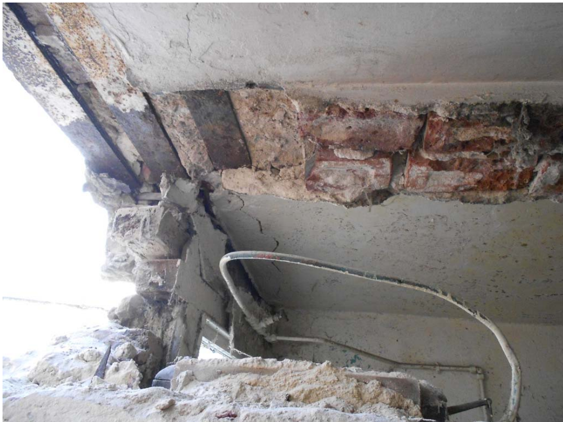
Photo 10: View of slab under kitchen. In a state of disrepair, currently being rebuilt by the Mohidiens.
