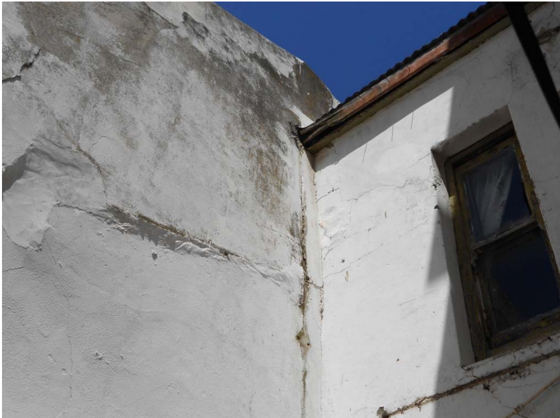
Photo 14: View inside back yard of barber shop. Note bad state of boundary wall.
