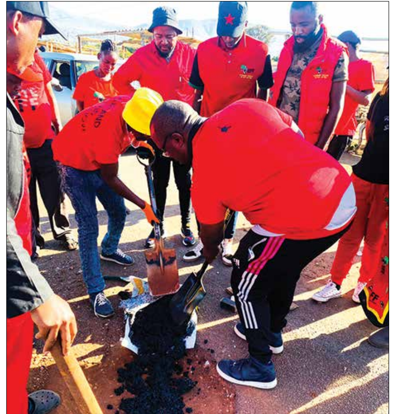
EFF Sekhukhune Region fixing potholes on the R37 Road around the Schoonoord area outside Jane Furse.
