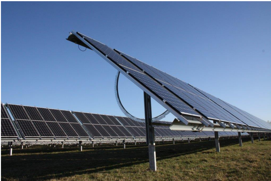
Figure 10: A view of installed single access tracking structures
