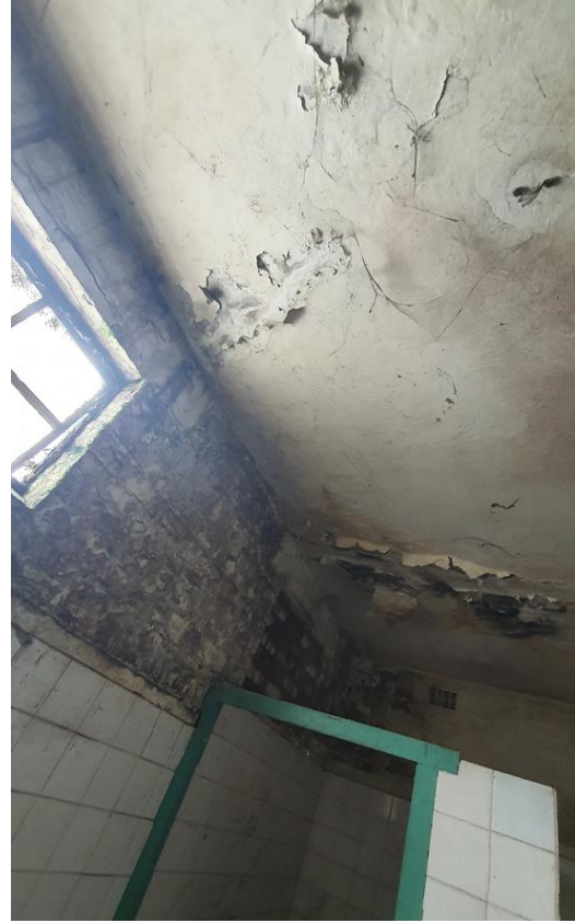
First Floor Ablution. Note water damage.
