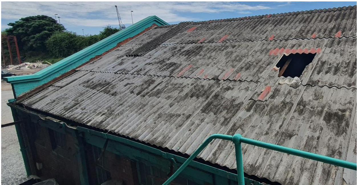
Roof damage to Building A
