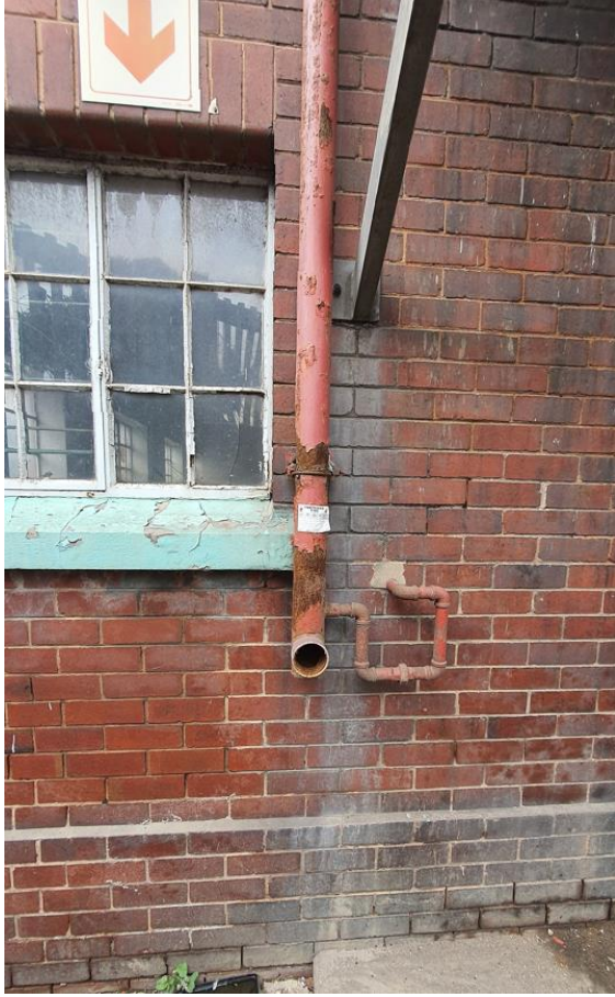
Redundant Fire Services
