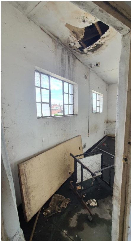
Third Floor water damage
