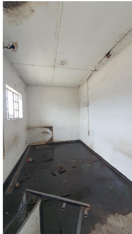
Third Floor water damage
