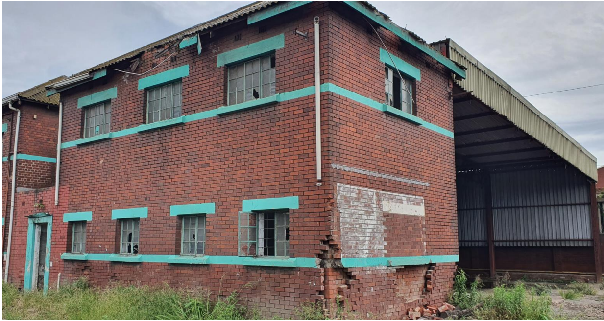
Damage to the North East corner
