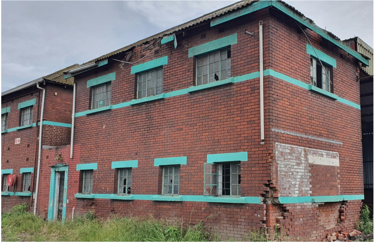
Structural Damage are evident to Building D to the North.
