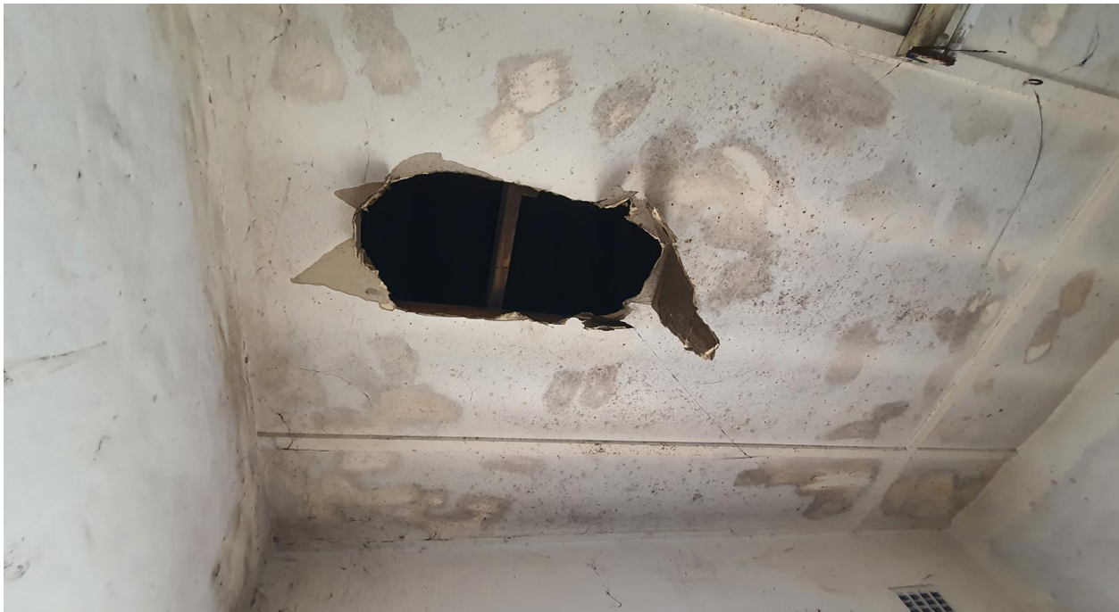
General Ceiling Damage
