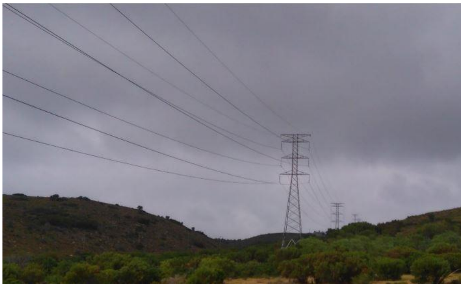
Figure 5: Example of a 132 kV transmission line
